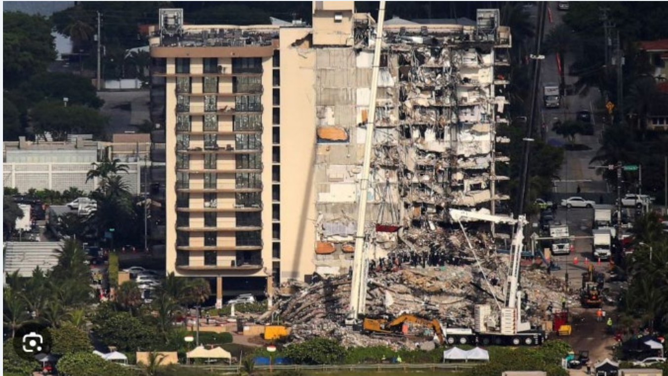
Champlain Towers South, 12-story condominium, Town of Surfside, FL June 24, 2021
