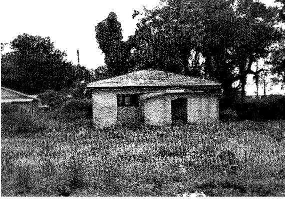
Dilapidated property on 10 th Court north of 79 th Street with worn paint and caved roof
