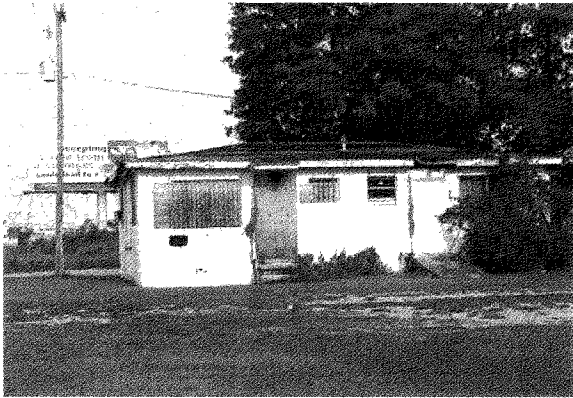
Dilapidated property 1205 79 th Street with boarded windows and defective roof
