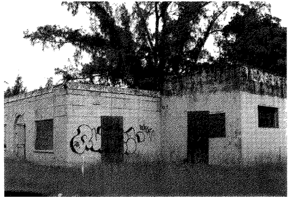
Dilapidated property on 79 th Street east of 17 th Avenue with graffiti, boarded windows and worn paint
