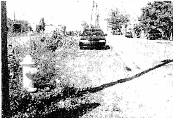
Roadway with missing sidewalk at NW 6 th Avenue and NW 20 th Street (Area A1)
