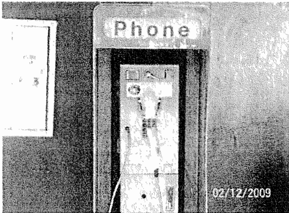
Damaged public fixtures (Area B2)
