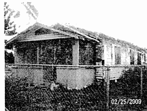
Vacant property at 570 NW 22 nd Street with significant structural damage, boarded windows, and damaged roof; built in 1924 (Area A1 east of I-95)
