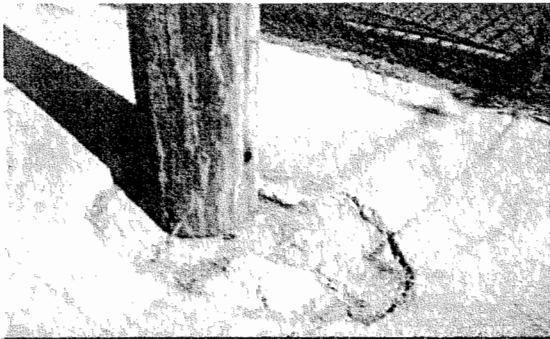
Improperly sealed utility pole (Area B2)
