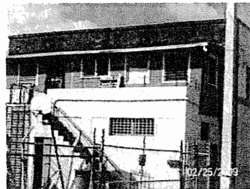
Property at 2195 NW 7 th Avenue with damaged roof and siding. (Area A1 west of I-95)
