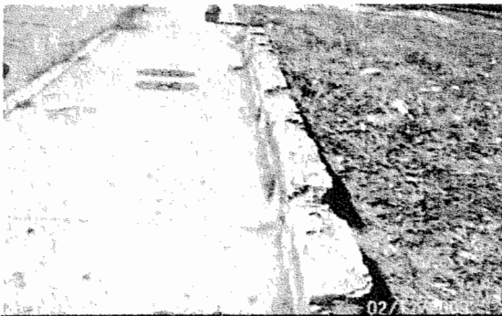
Incomplete site cleanup after demolition (Area B2)
