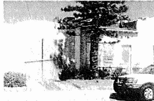
Property at 521 NW 7 th Street with boarded garage and peeling paint; built in 1920 (Area B2)
