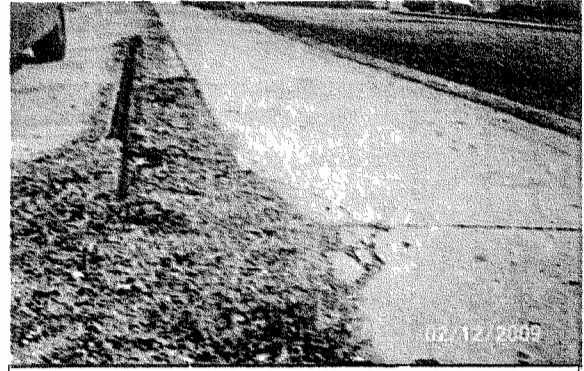
Foreign material protruding from ground (Area A1)
