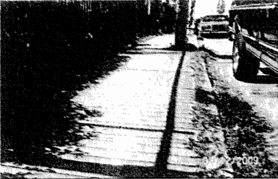
Lack of sidewalk maintenance (Area B2)
