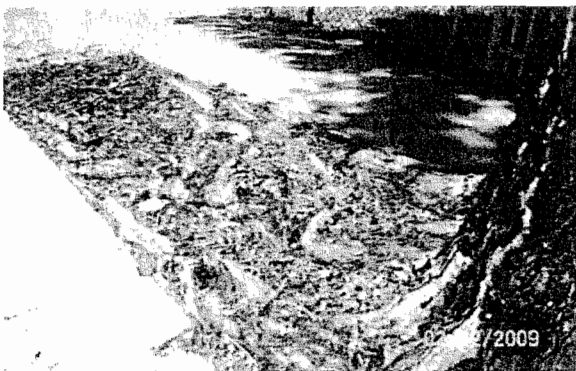
Missing sidewalk resulting from lack of tree maintenance (Area A1)
