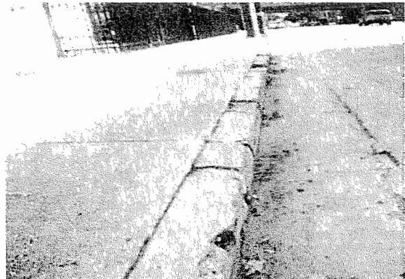
Chipped sidewalk, at NW 8 th Street between NW 3 rd Court and NW 4 th Avenue (Area B2)
