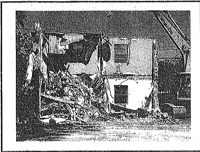
Unsafe Structure Demolition 6442 SW 59 th PL
