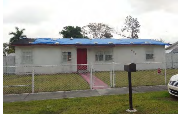
Figure 7: Unrepaired roofs pose a safety risk
