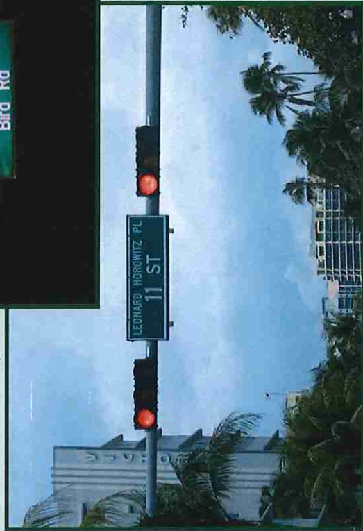
Illuminated Street Sign LED Traffic Lights
