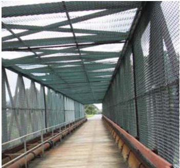
Utility lines interfere with trail width
