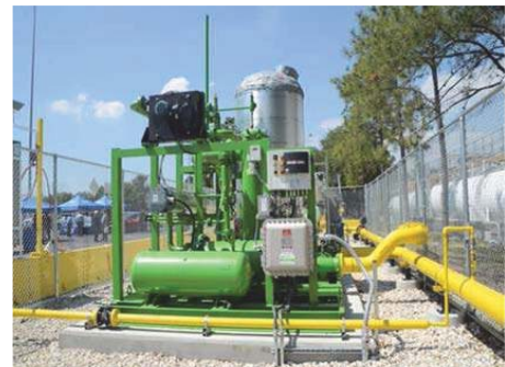
HART's CNG station is designed to fuel 250 buses.
