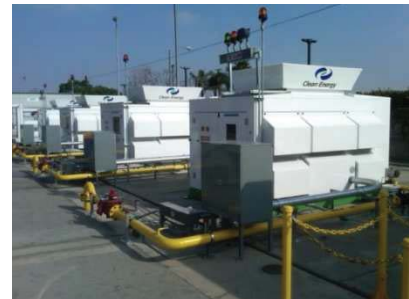
Clean Energy maintains all 10 LAMTA CNG stations.
