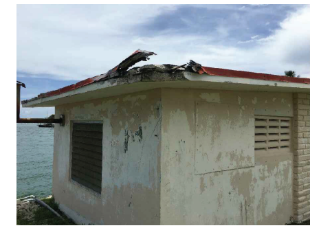
SPALL DAMAGE EXHIBIT (NE CORNER)
