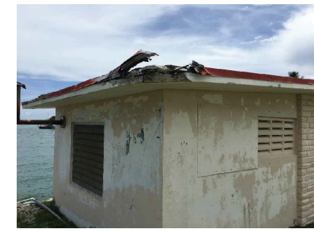
SPALL DAMAGE EXHIBIT (NE CORNER)
