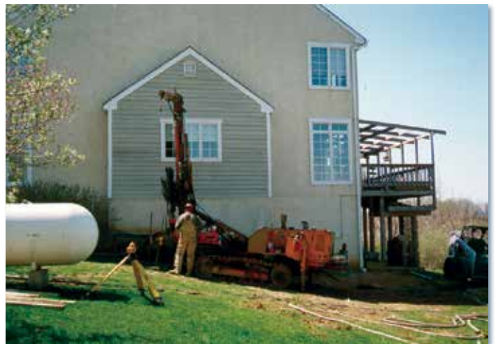
Compaction grouting was performed at interior and exterior locations, with minimal disturbance to townhouse residents.
