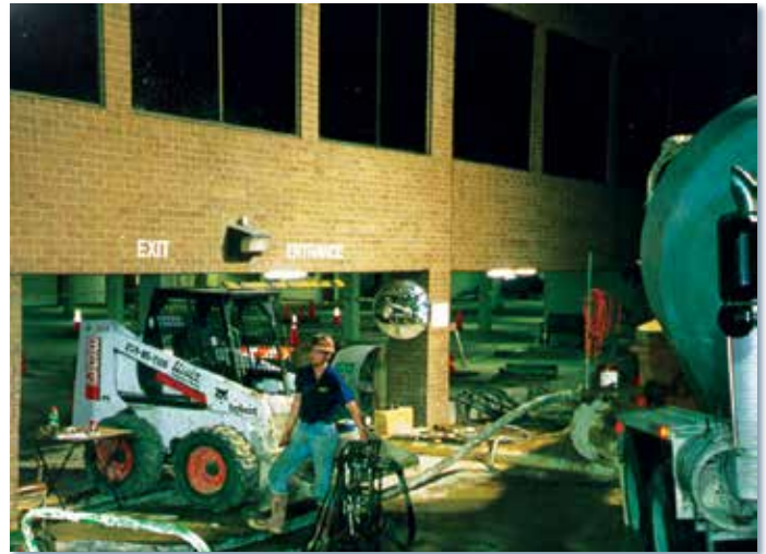
Compaction grouting stabilized the rubble fill underlying a four-story building and successfully restored the building to near original elevation.
