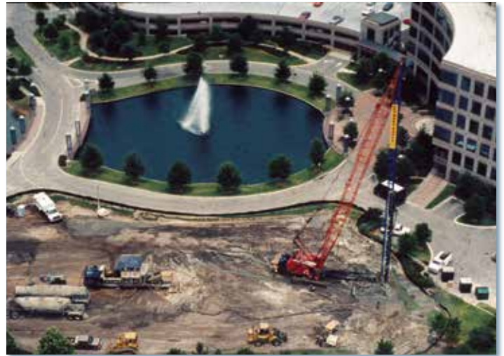
Compaction grouting to pre-treat the Summit site reduced the risk of future sinkhole activity.
