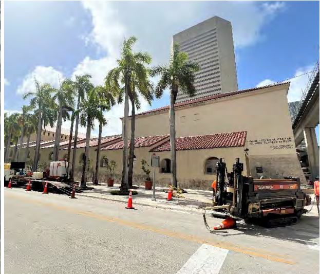
Looking Northwest from W Flagler Street toward the southeast entrance to the Cultural Center Block
