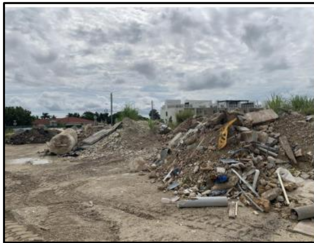
Debris piles during construction
