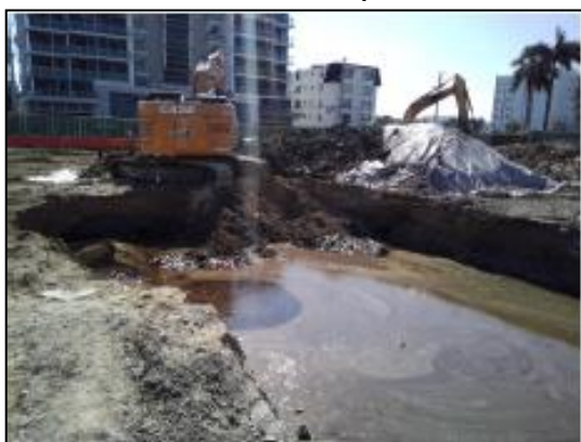
Excavation with free floating product
