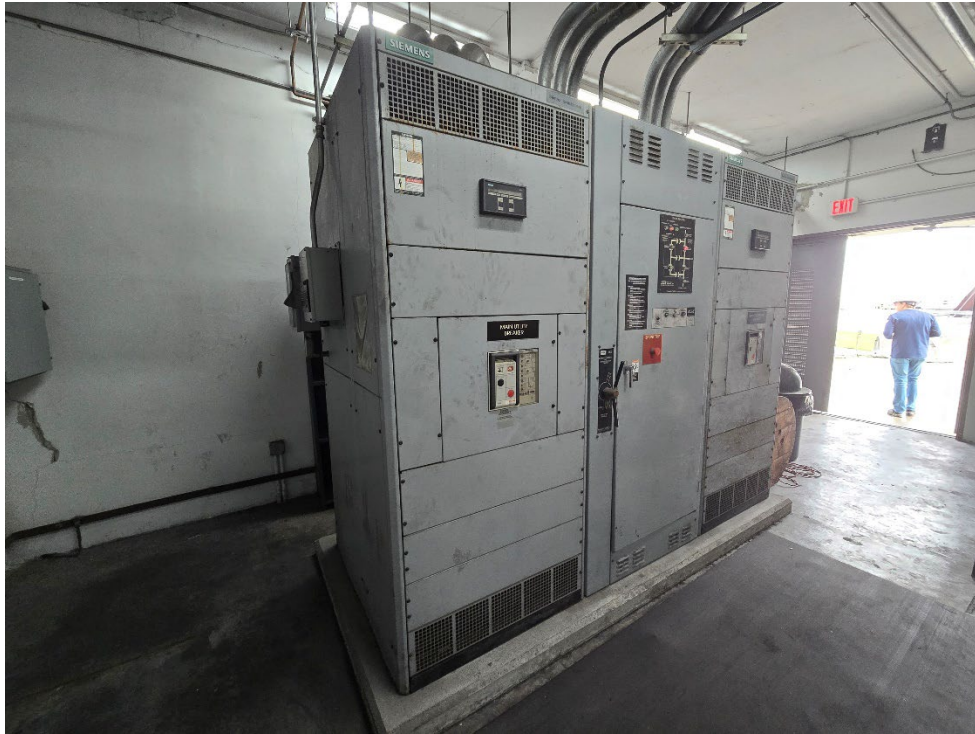
Figure 1.4 – Switchgear with entry doors in rear
