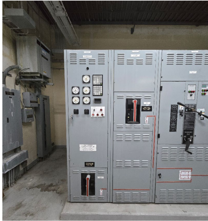
Figure 2.15 – Side photo of switchgear associated with 900 KW generator (this unit to be replaced)
