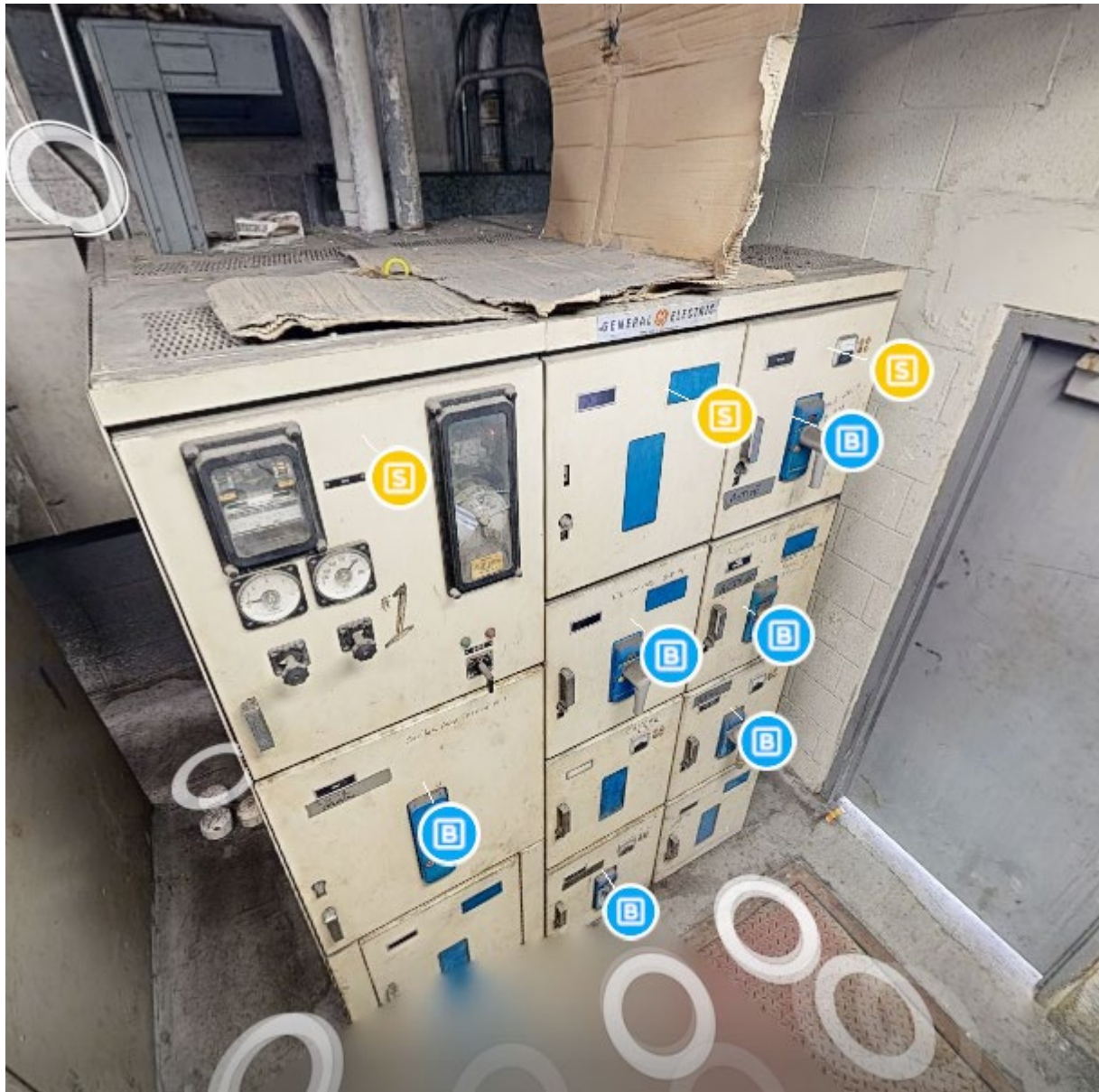
Figure 3.9 – Matterport image of MDS #1. Active panels present include loads to interior terminal & chiller.
