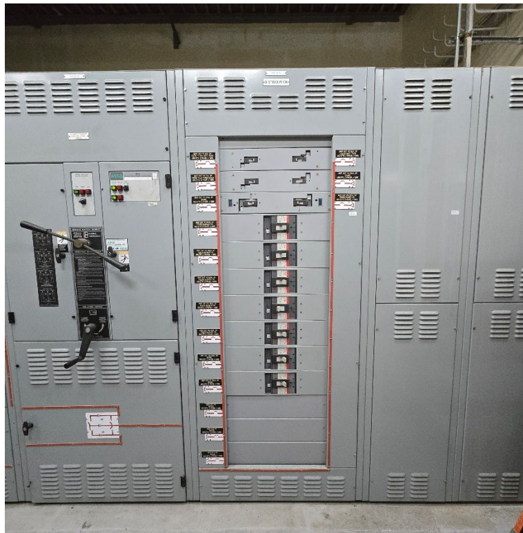
Figure 2.16 – Side photo of switchgear associated with 900 KW generator (this unit to be replaced)
