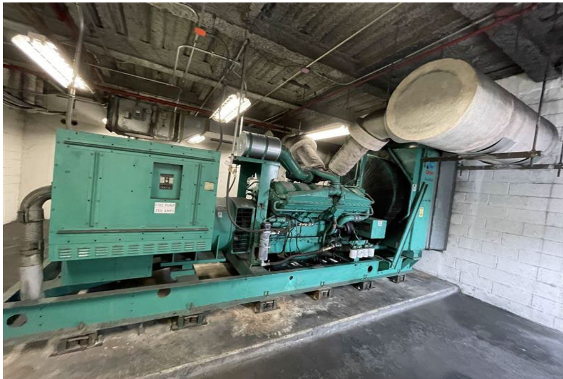
Figure 2.3 – Frontal view of generator (North side)
