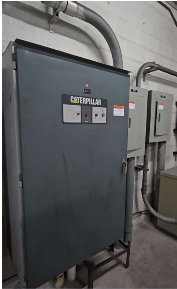
Figure 5.13 – ATS #1 on south wall of switchgear room with associated emergency panel to left of photo. Located directly behind & downstream of main panel in figure 3, on other side of wall.
