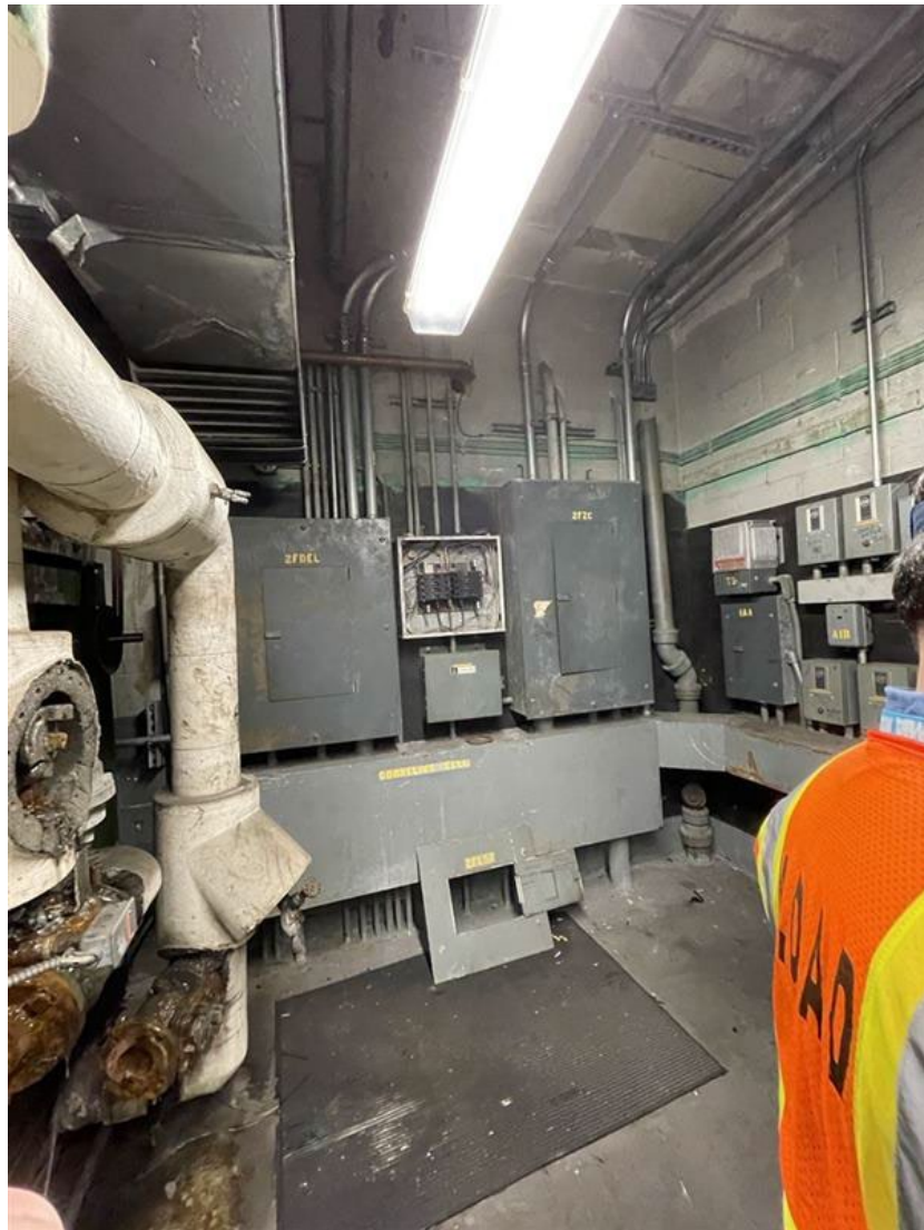
Figure 3.18 – Subpanels in mechanical room 1829
