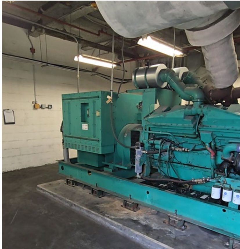
Figure 3.4 – Alternative frontal view of generator taken from doors (east wall in back)
