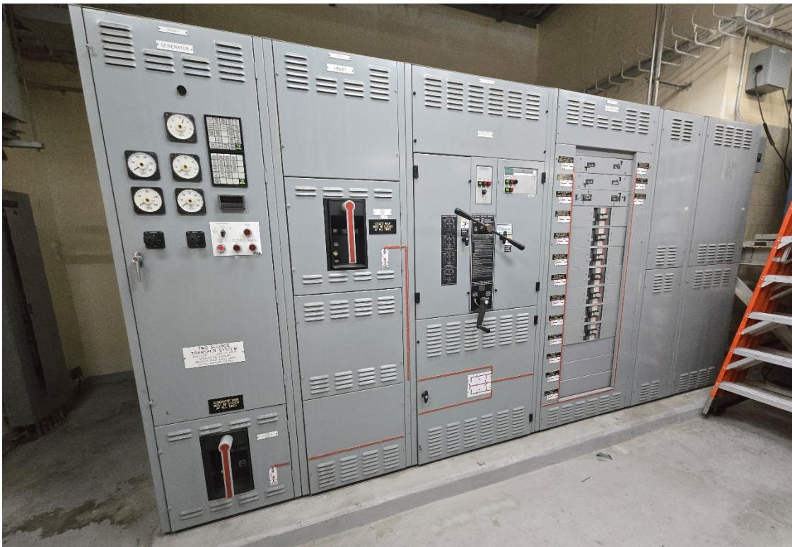
Figure 2.14 – Switchgear unit in lighting room, associated with 900 KW generator (this unit to be replaced)
