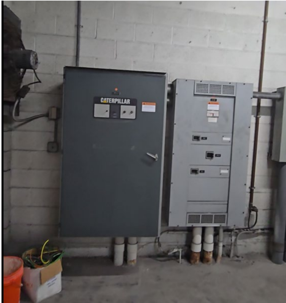
Figure 5.12 – ATS #2 on south wall of switchgear room with associated emergency panel. Located behind Switchgear #2. Downstream of pipes shooting to right from main panel in Figure 5.2 (on other side of wall).
