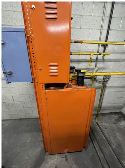
Figure 5.6 – Side view of diesel day tank
