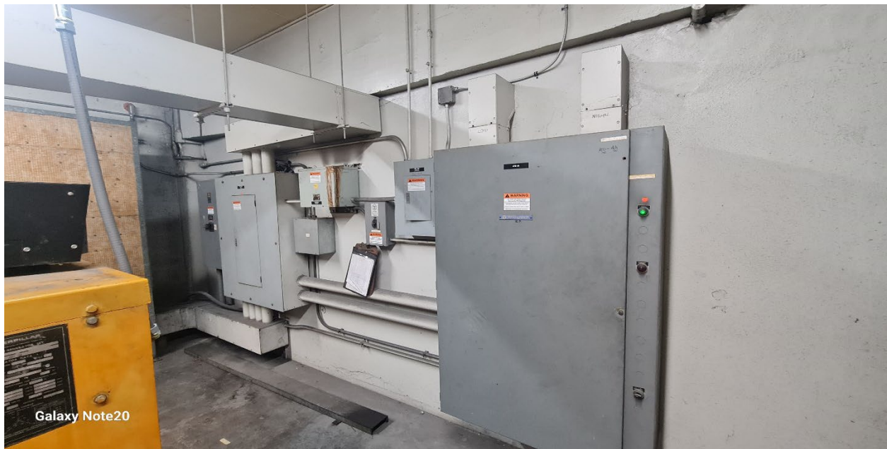
Figure 4.5 – North wall of generator room. Includes 2 ATS's and main duct from generator. Adequate space.
