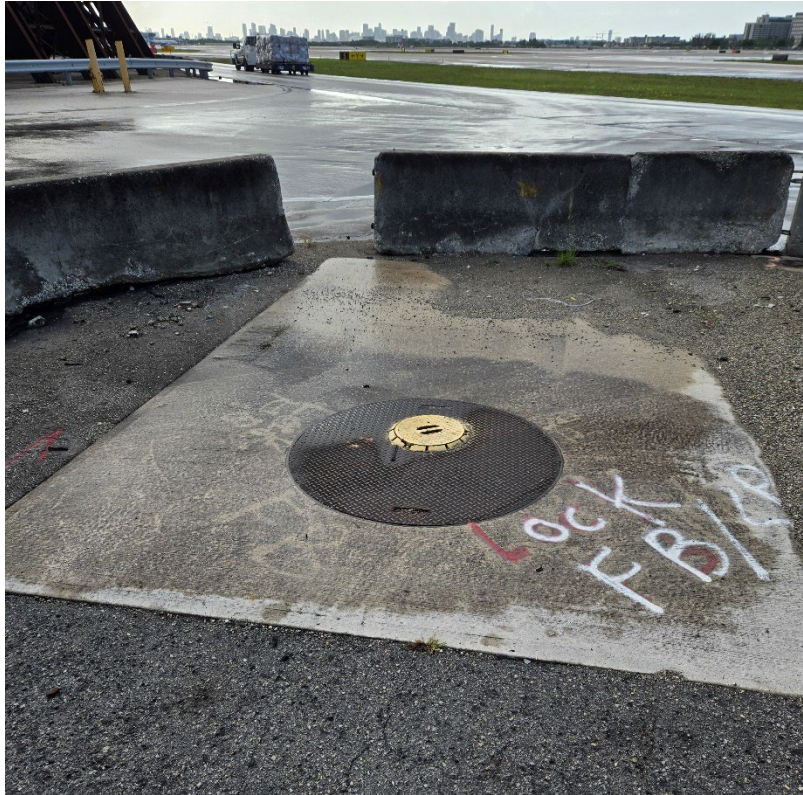
Figure 1.12 – Underground diesel storage tank location (~85ft SE of pad mounted transformer)
