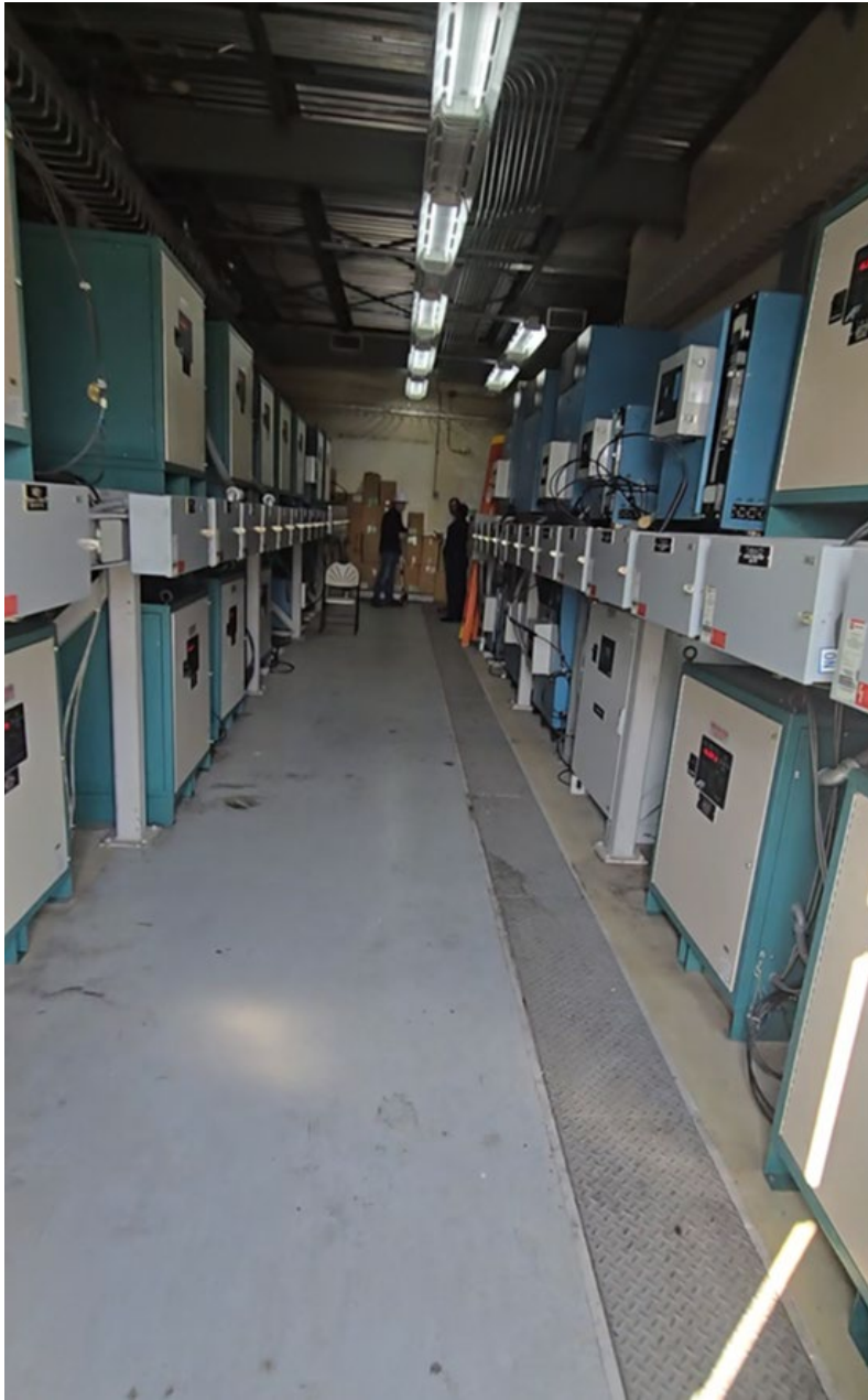
Figure 2.18 – Lighting room “regulator room” hallway leading to switchgear unit at end of hall on right, taken from entry doors
