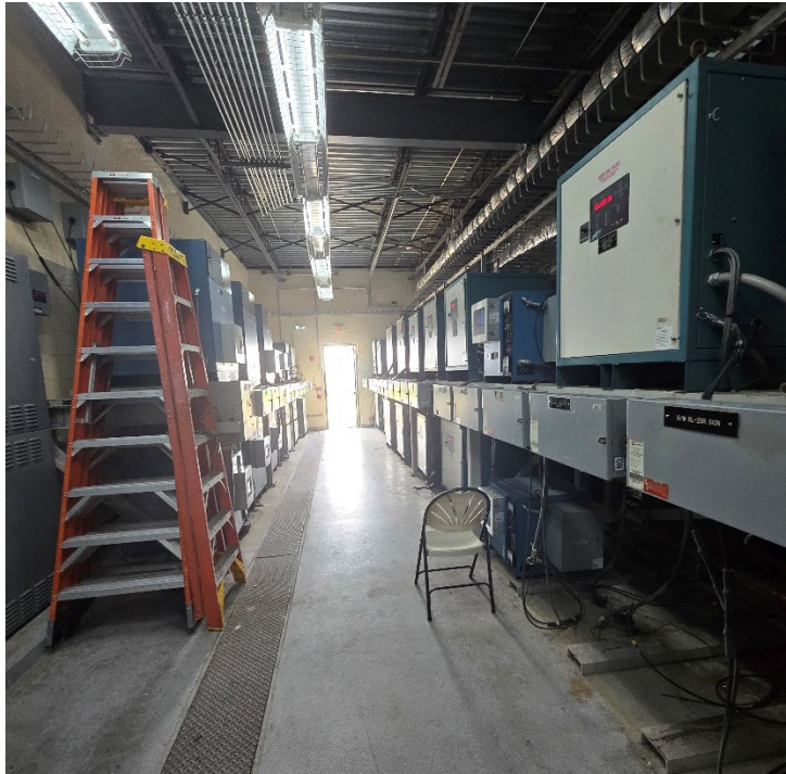
Figure 2.17 – Lighting room hallway leading to entry doors, taken from 900KW gen associated-switchgear unit
