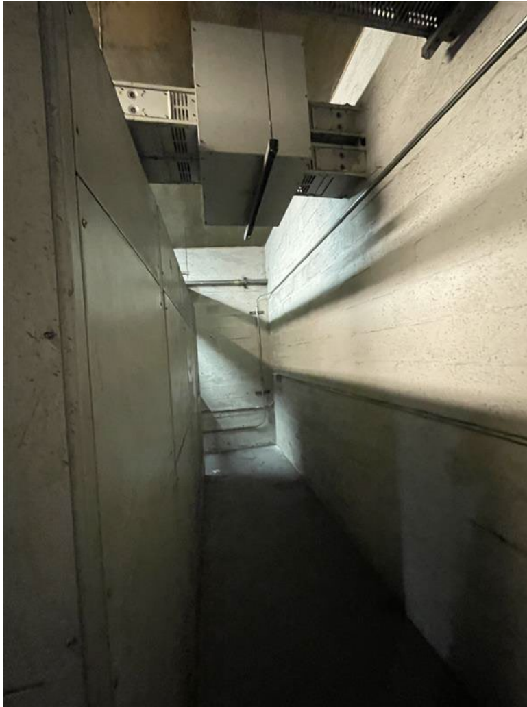
Figure 4.10 – Rear side of switchgear with overhead bus duct leading to FPL vault thru north wall
