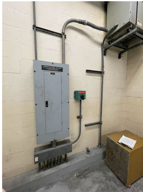
Figure 2.12 – Northwest corner of 900KW Generator Room
