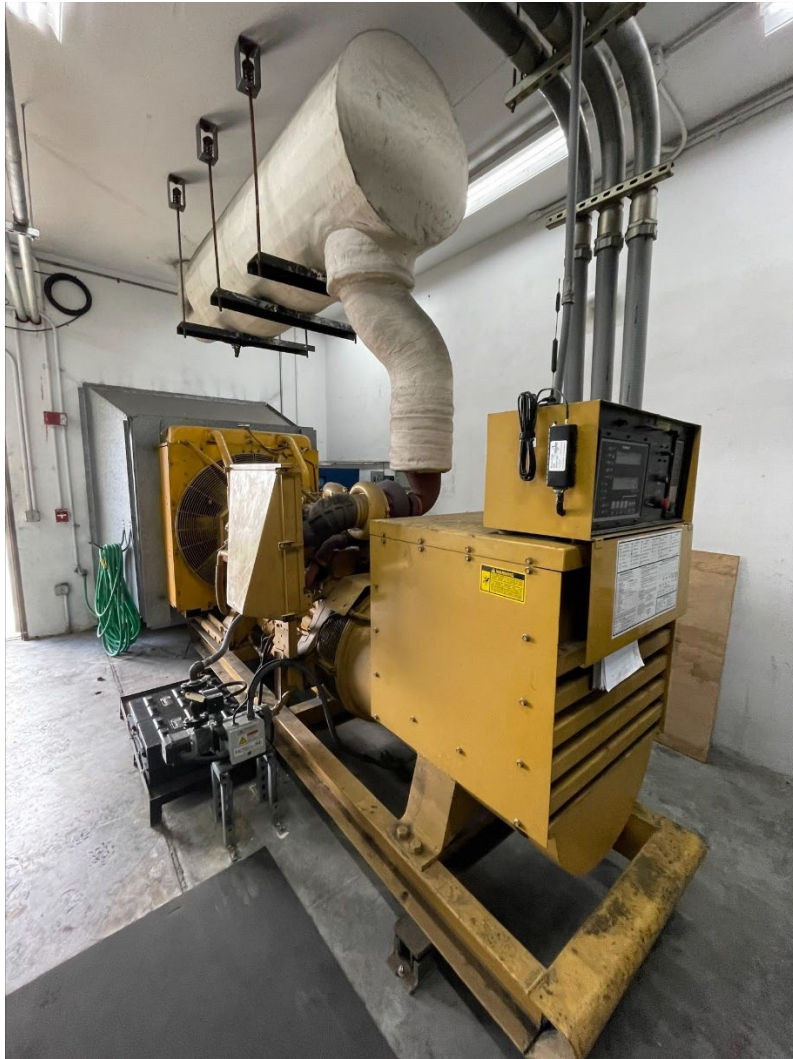
Figure 1.5 – Angled view of generator
