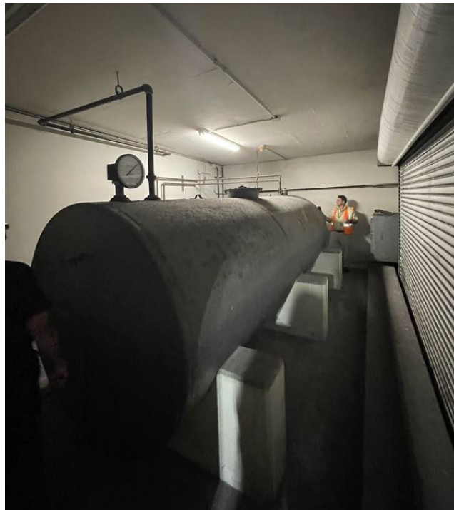
Figure 4.18 – 2400-gallon diesel tank
