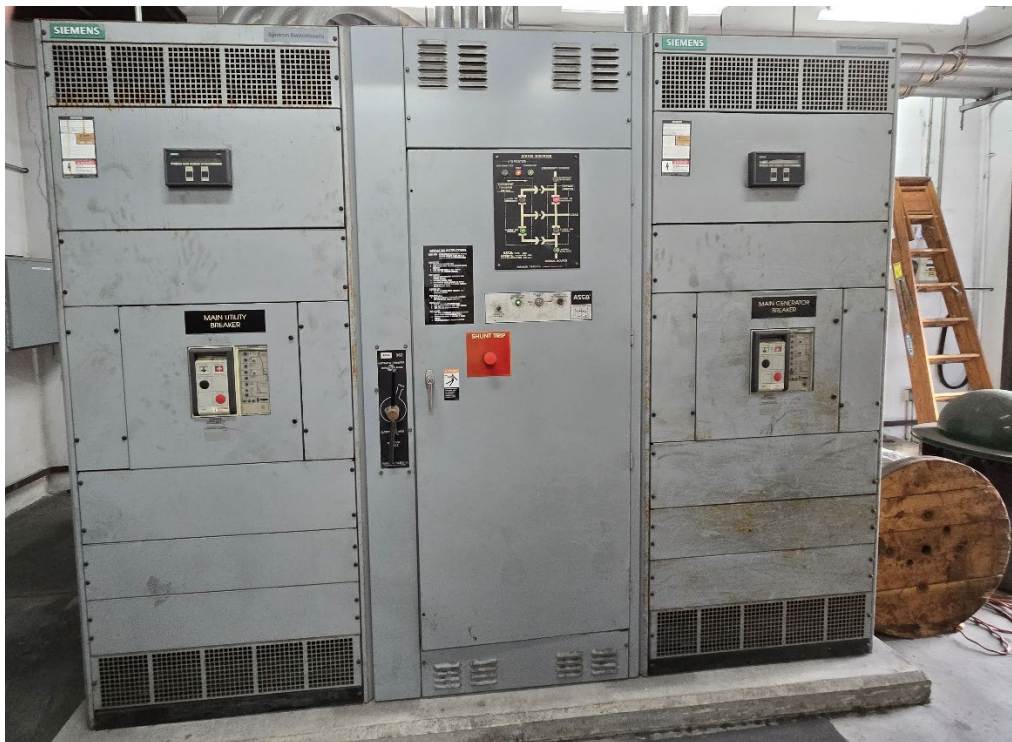
Figure 1.3 – Frontal view of switchgear
