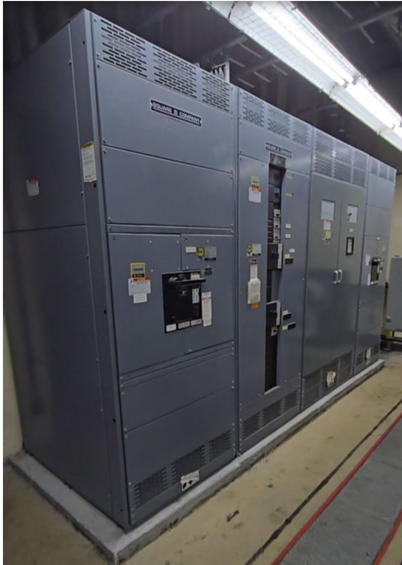
Figure 2.6 – Switchgear unit to remain as-is (associated with 500 KW generator). Located outside of generator room(s).
