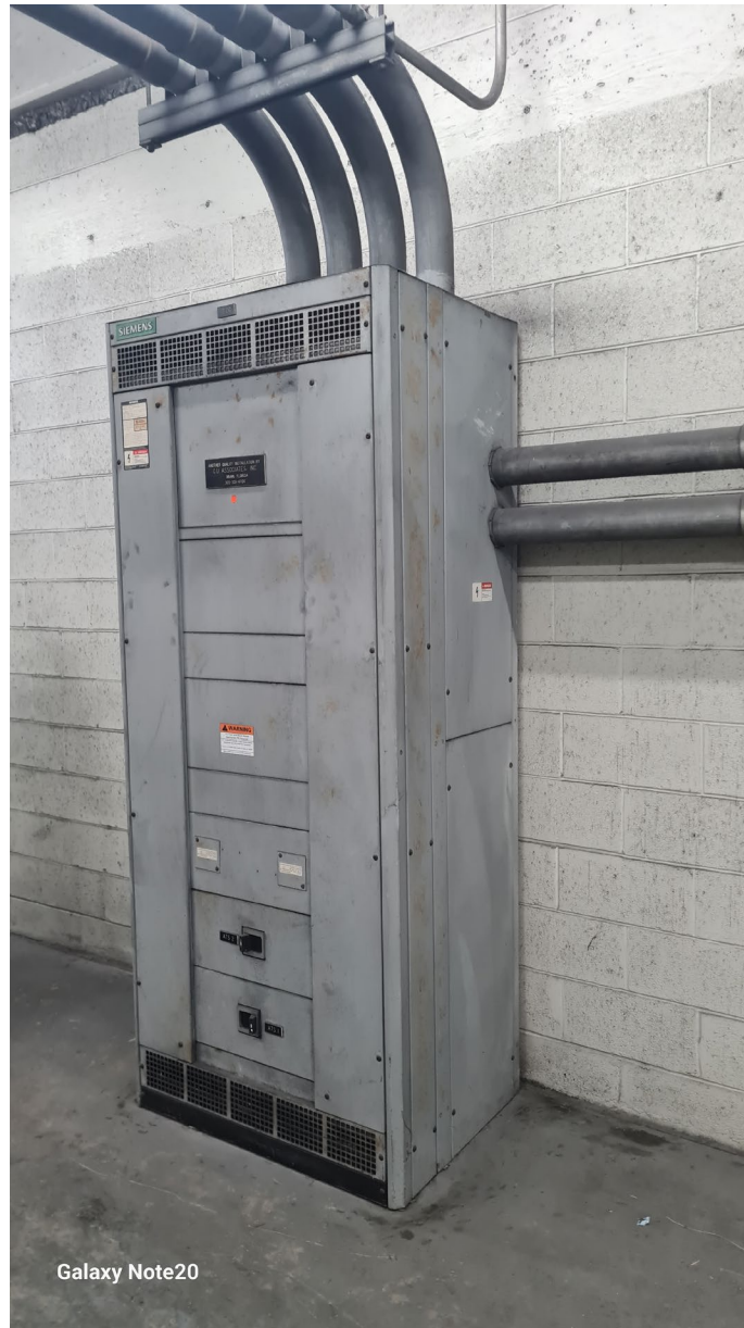
Figure 5.7 – Immediate downstream panel from generator, receiving 4 overhead pipes. Plans indicate cable size of (4) 500MCM. 2 ATS outputs are on other side of wall.
