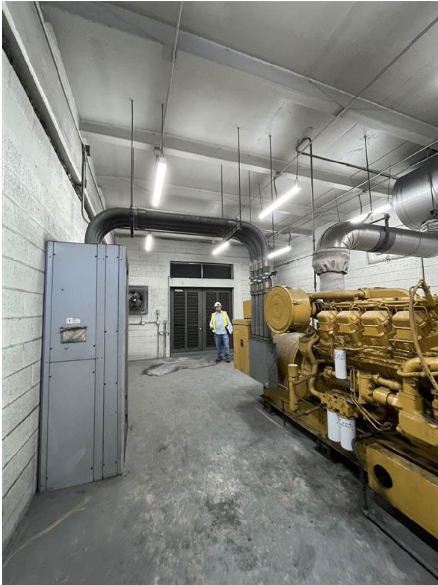
Figure 5.4 – Alternate view of generator room. East doors to room in rear of photo.
