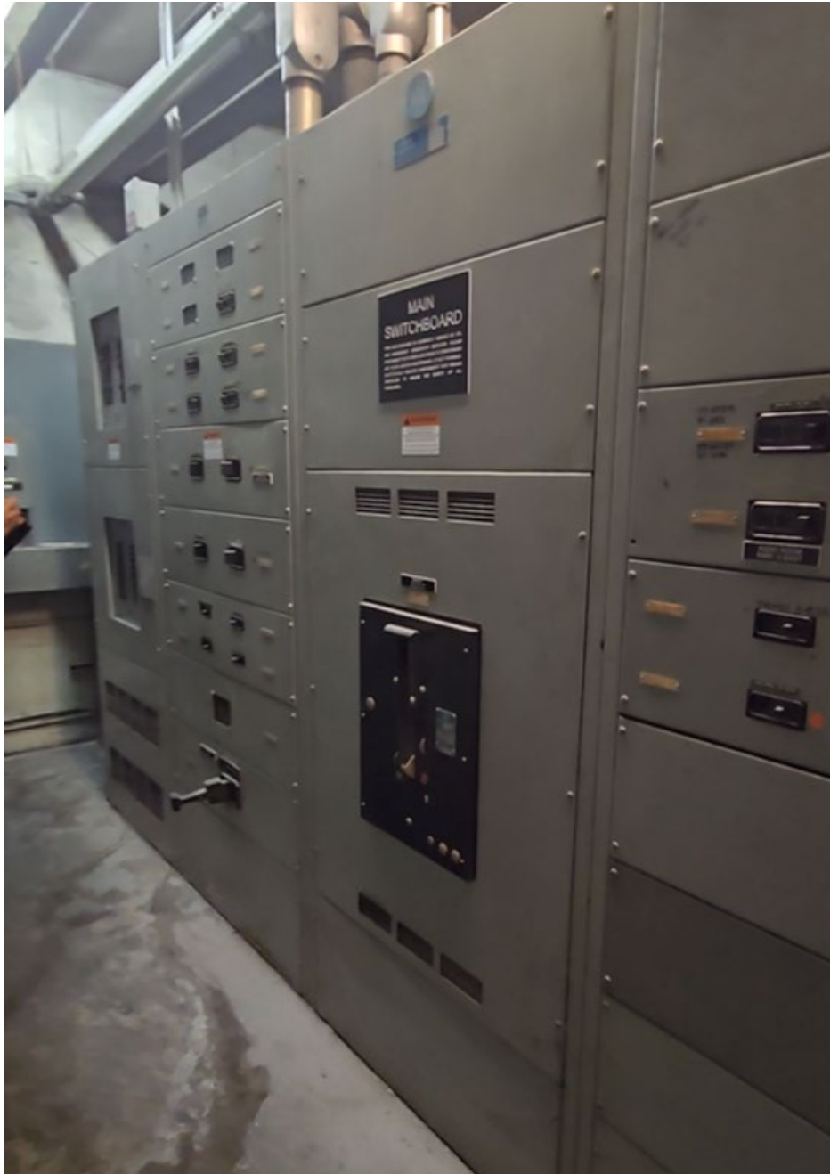
Figure 4.8 – Angled view of the switchgear
