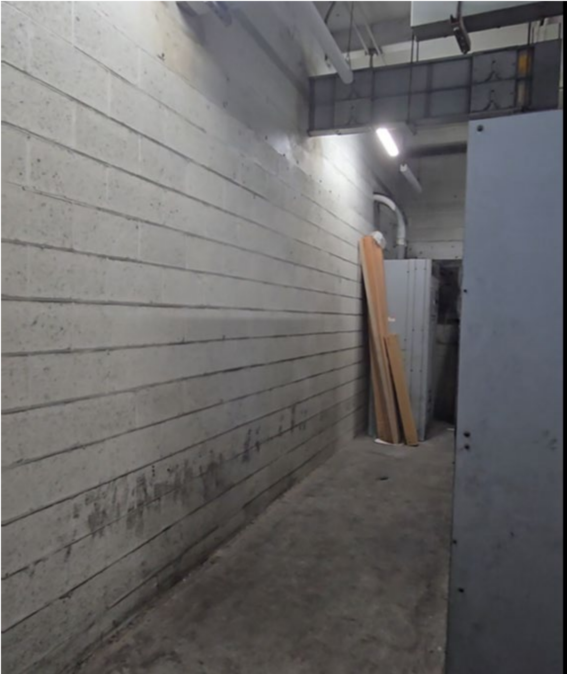
Figure 5.14 – Space behind Switchgear #1 & north wall (~4-5ft of space). FPL vault located behind wall.
