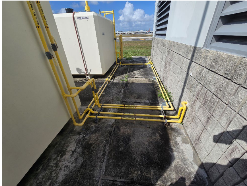
Figure 2.19 – Diesel pipes running into bldg. from twin 4000-gal diesel tanks
