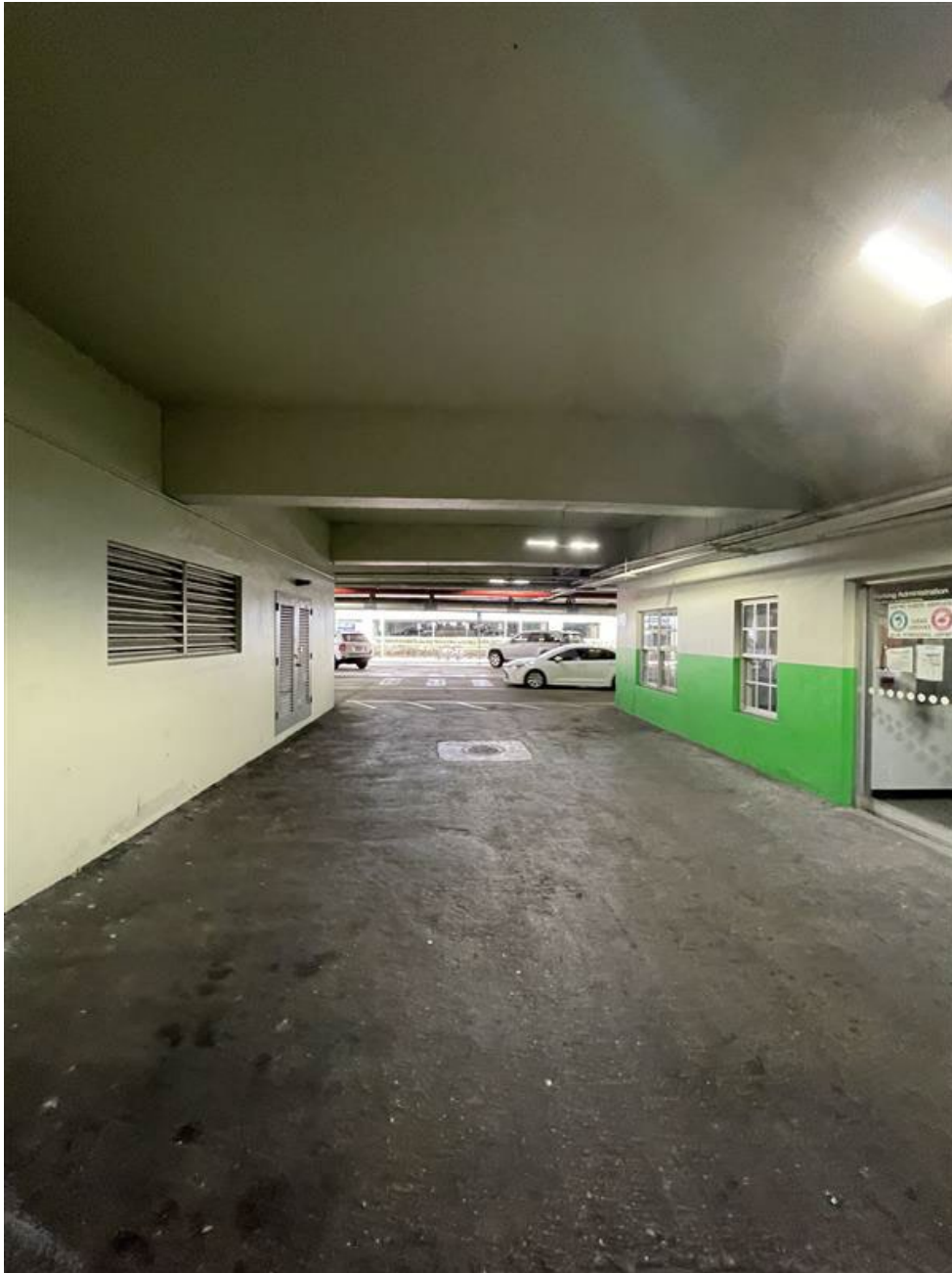
Figure 4.11 – Hallway leading to generator and electrical rooms - facing north. Parking lot and outdoor road located in rear of photo. The FPL vault doors are visible on left side of photo. Generator and electrical rooms lie directly to left of photo.
