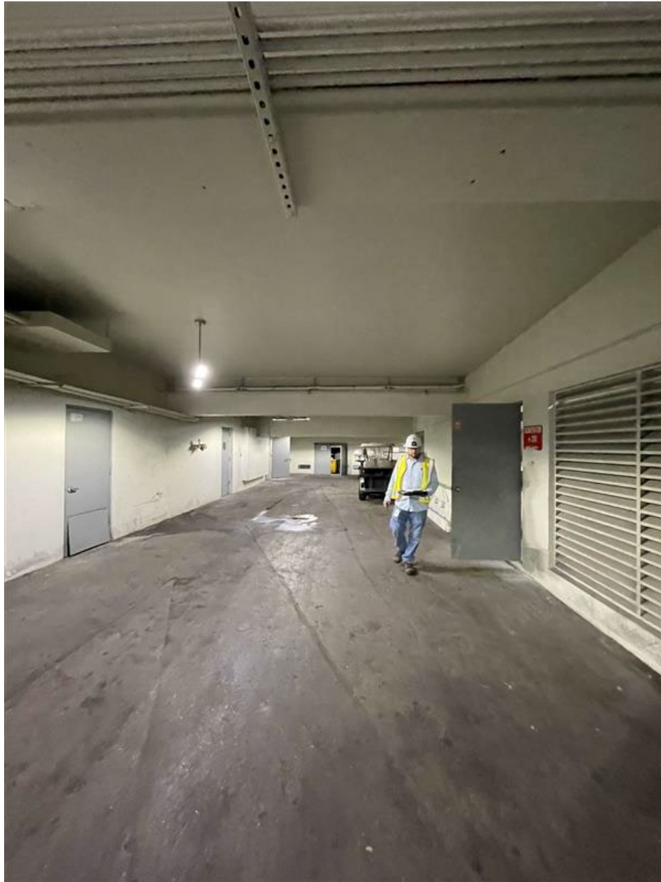
Figure 4.12 – Hallway leading to electrical room and generator room, facing south. The electrical room is the open door on right side of photo.
