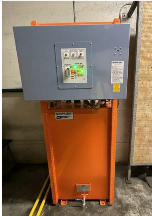
Figure 4.4 – Day tank in generator room
