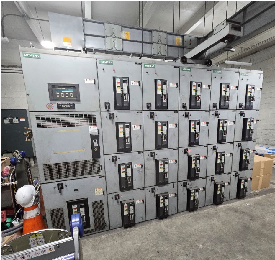
Figure 5.11 – Alternate view of south switchgear (Switchgear #2)
