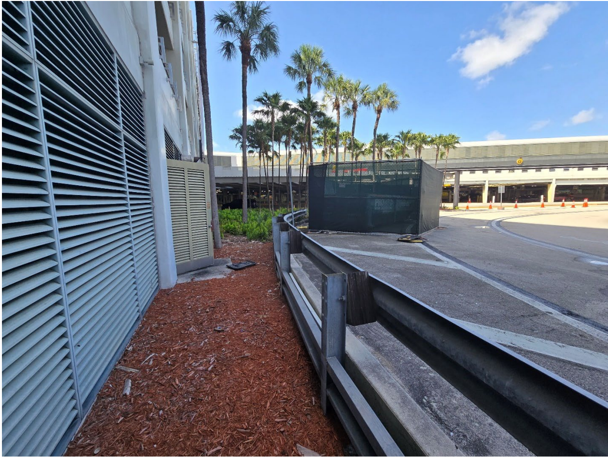
Figure 5.19 – Location outside of generator and switchgear rooms, taken roughly 25ft north of Figure 19 in same direction.
