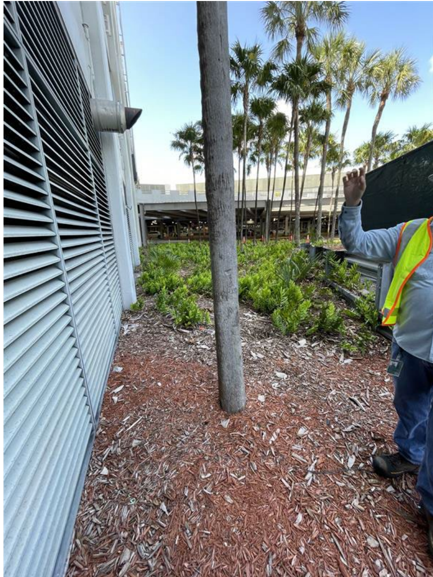
Figure 5.18 – Mulch/trees/bushes outside of electrical and switchgear rooms. Road and dumpster to right of photo. Potential landing area for temporary equipment and general construction access. Photo faces south from switchgear room doors.
