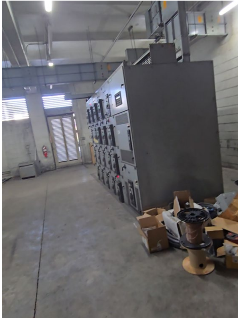
Figure 5.8 – “North” switchgear unit #1 in switchgear room, taken from main door. Bus duct enters FPL vault behind photo to right.
