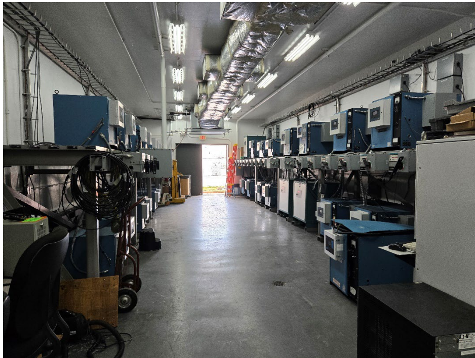
Figure 1.8 – Lighting room in rear of building. Temporary conductor route to be placed along floor from outdoor entry.
