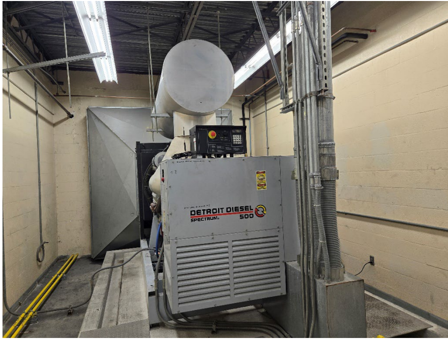
Figure 2.2 – 500 KW Generator Room (looking in from door)
