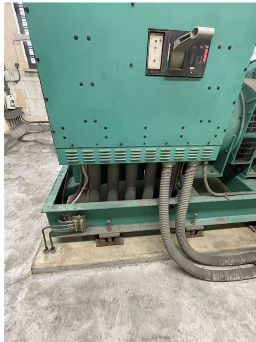
Figure 2.10 – 900 KW Generator's downstream conductors
