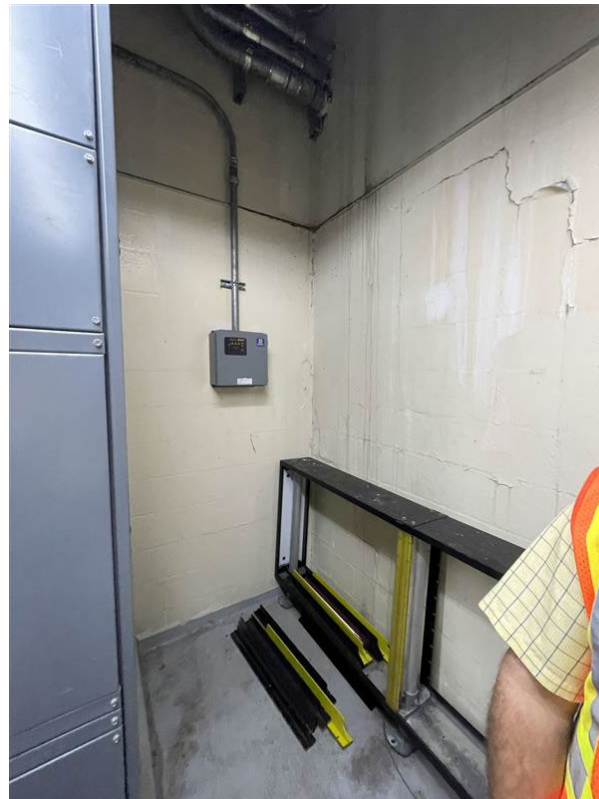
Figure 2.7 – Space to right of 500 KW-associated switchgear unit
