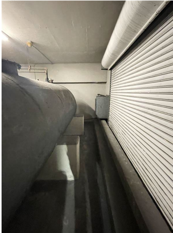
Figure 5.20 – Frontal view of 2600-gallon diesel tank
