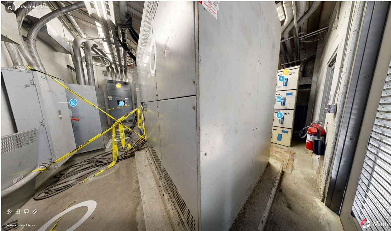
Figure 3.14 – Matterport image POV from NW corner. Switchboard DPMG, exposed cables, temporary feeder panels, located in rear of Substation Mains #1 and #2. Exterior doors to room on right side of image. Roughly 3ft clearance between Switchboards and left (North) wall.
