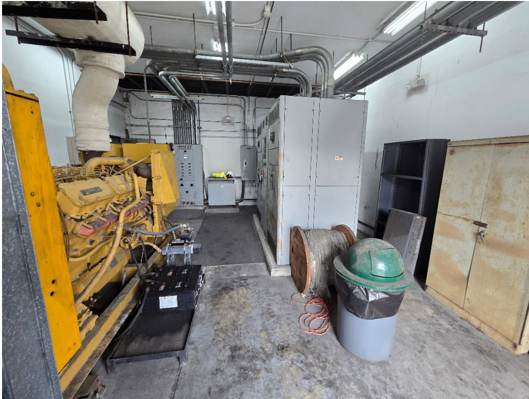
Figure 1.2 – Electrical/generator room, from POV at main entry doors. Generator on left, switchgear on center-right, and MDP located in rear-left. Utility feed entering overhead from top right of photo.
