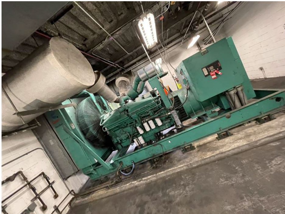
Figure 3.5 – Back view of generator (south side)
