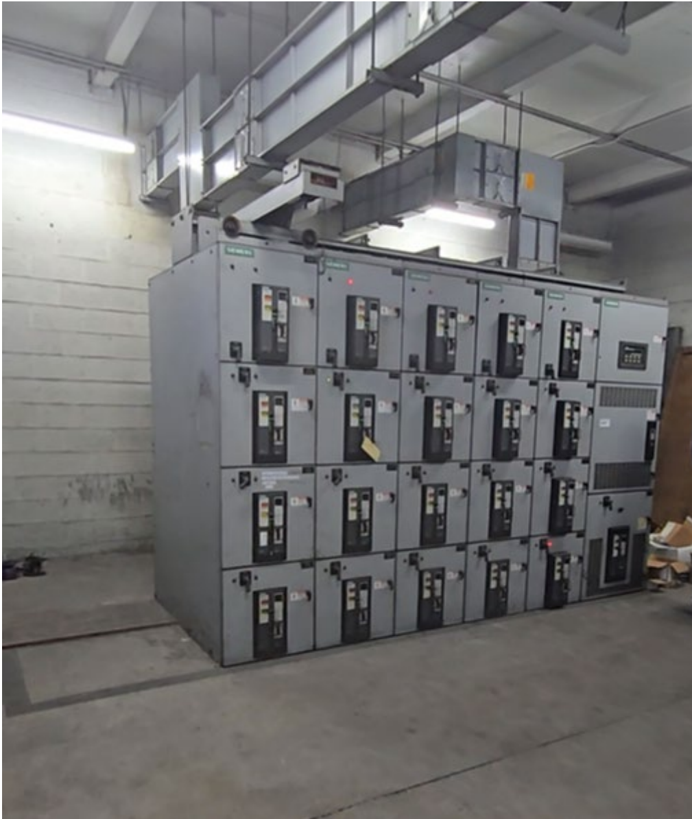
Figure 5.9 – Alternate view of north switchgear unit (Switchgear #1)
