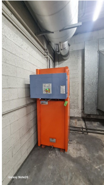
Figure 5.5 – Diesel Day tank in generator room
