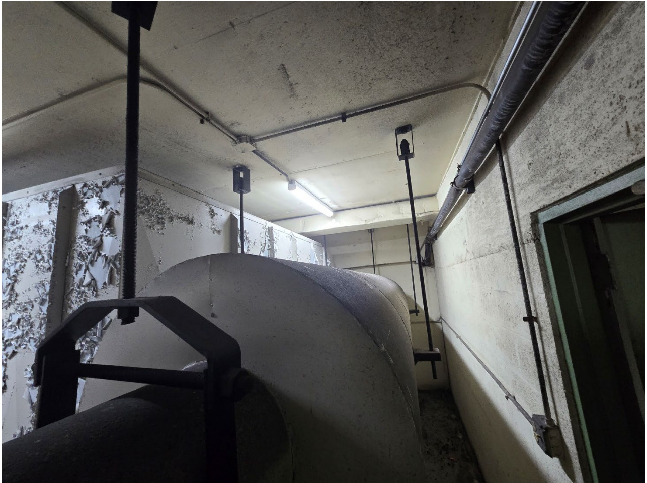
Figure 4.13 – Exhaust room view facing north towards generator.
