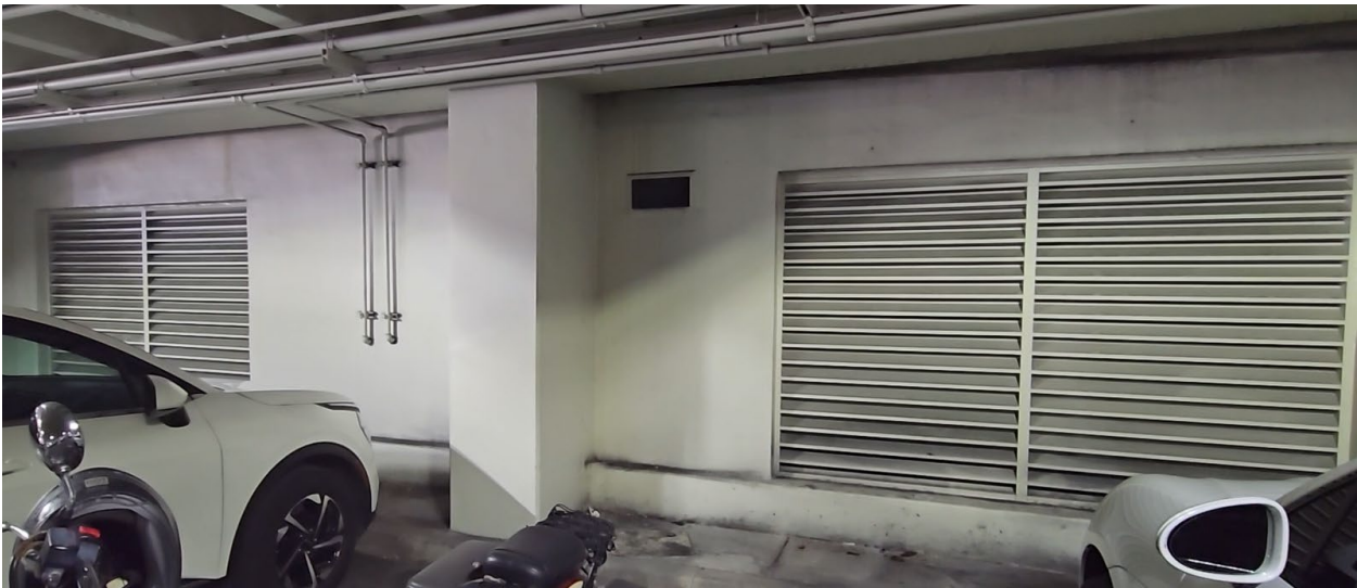
Figure 4.15 – Rear side (west) of electrical/generator rooms. Left plenum is air intake for generator and right plenum is associated with radiator exhaust system (ref figures 10 & 11).
