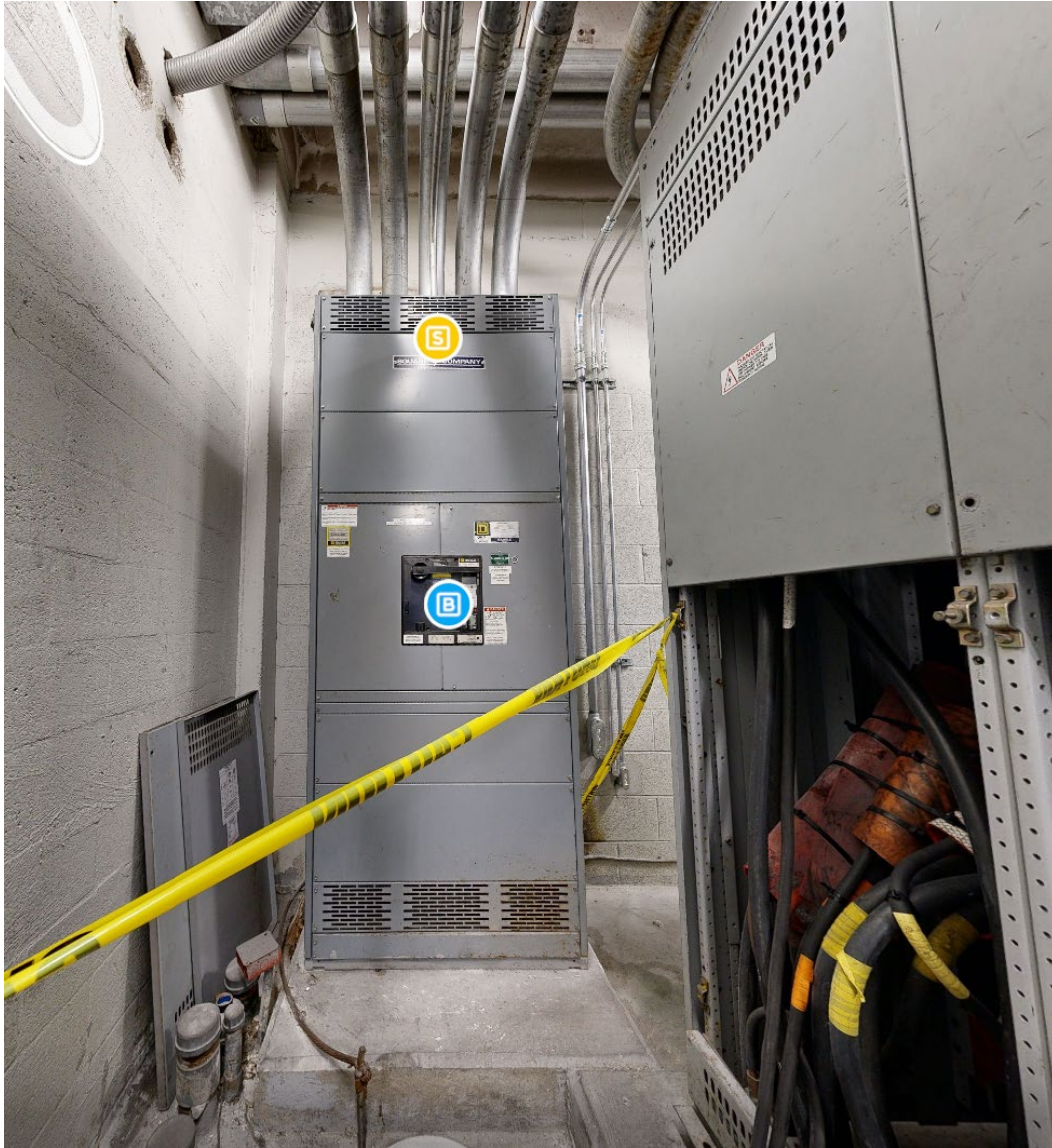
Figure 3.13 – Matterport image of Switchboard DPMG, located in NE corner of room. Caution tape and panel boards missing in rear of Substation Main #2, with exposed cable. Take heavy caution.
