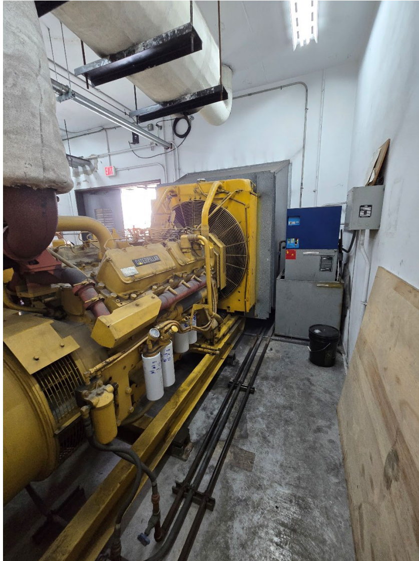
Figure 1.6 – Rear view of generator with diesel day tank in corner. Main entry doors to room visible behind generator
