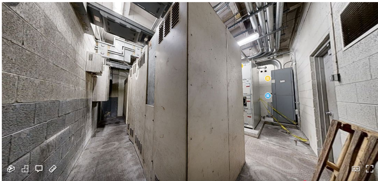
Figure 3.12 – Matterport Image POV from SE corner. MDS#2 in front. Roughly 3ft clearance between MDS#2 and south wall. Mechanical room door visible on right with Switchboard DPMG in rear right. FPL vault located behind left (south) wall.
