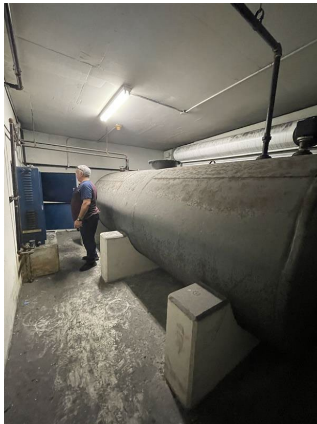
Figure 4.19 – 2400-gallon diesel tank
