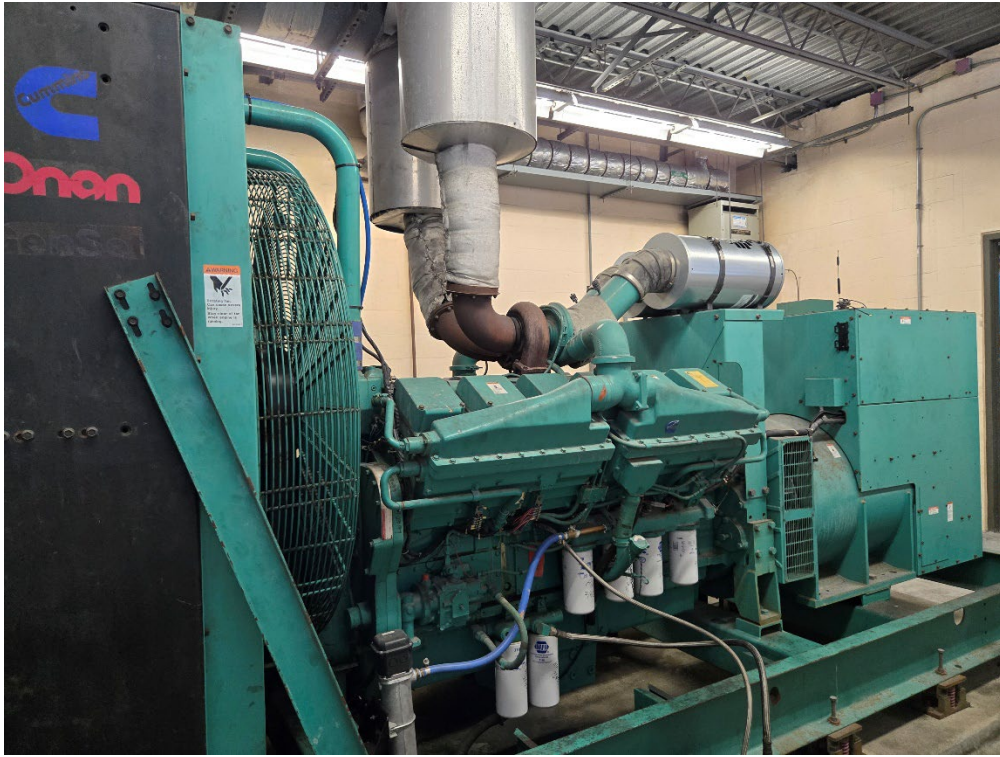
Figure 2.9 – Angled view of 900 KW generator
