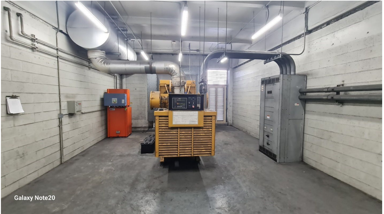
Figure 5.2 – Generator room – taken from main doors on east wall.
