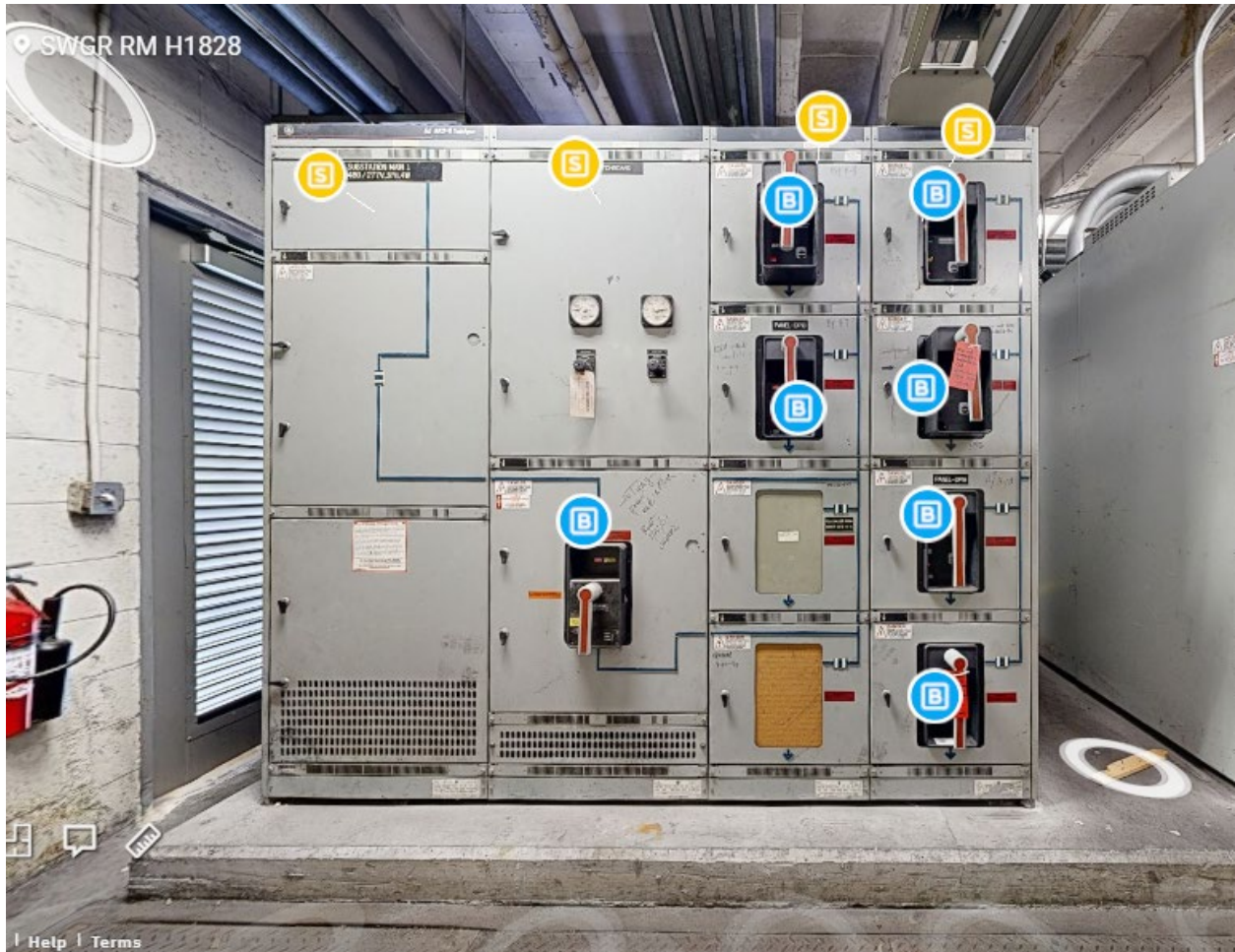
Figure 3.8 – Matterport image of Substation Main #1. 4 main sections across the top. Several panels present including jetway and chiller loads.
