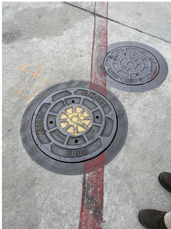
Figure 3.17 – Underground diesel storage tank location (outside of generator/electrical rooms)
