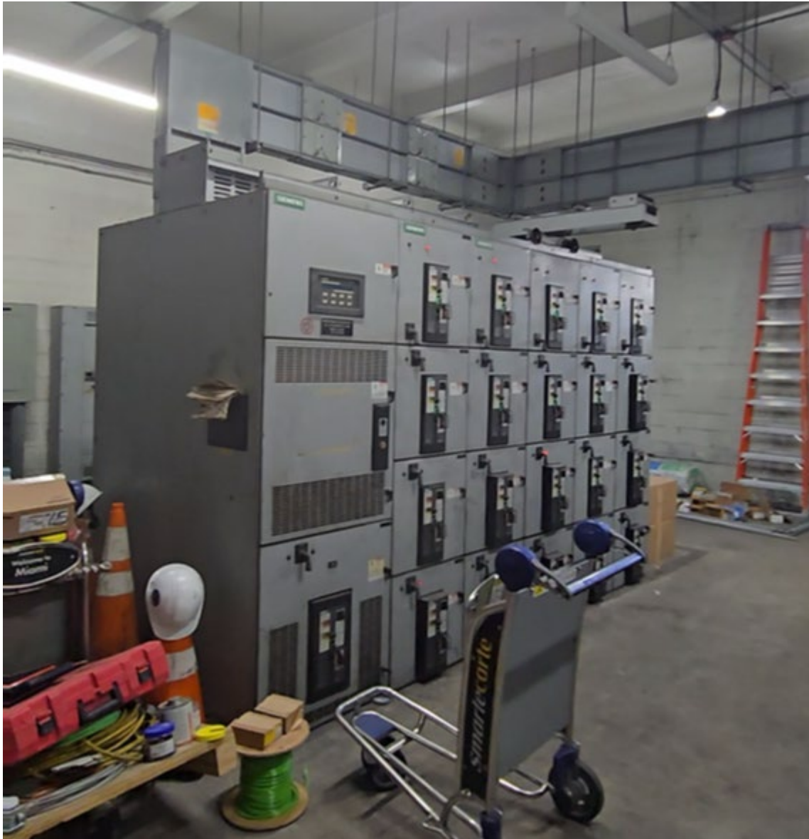
Figure 5.10 – “South” switchgear, taken from room’s main doors (Switchgear #2)
