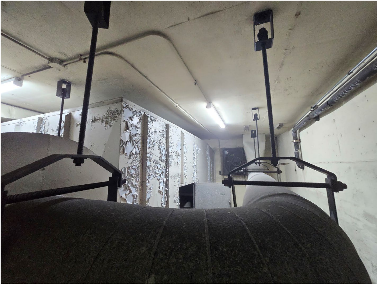
Figure 4.14 – Exhaust room view facing west. Exhaust system turns upwards in background towards top of garage.
