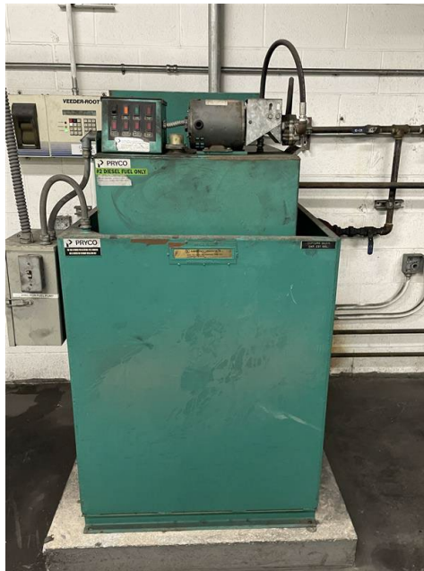
Figure 3.6 – Diesel day tank in SW corner of generator room
