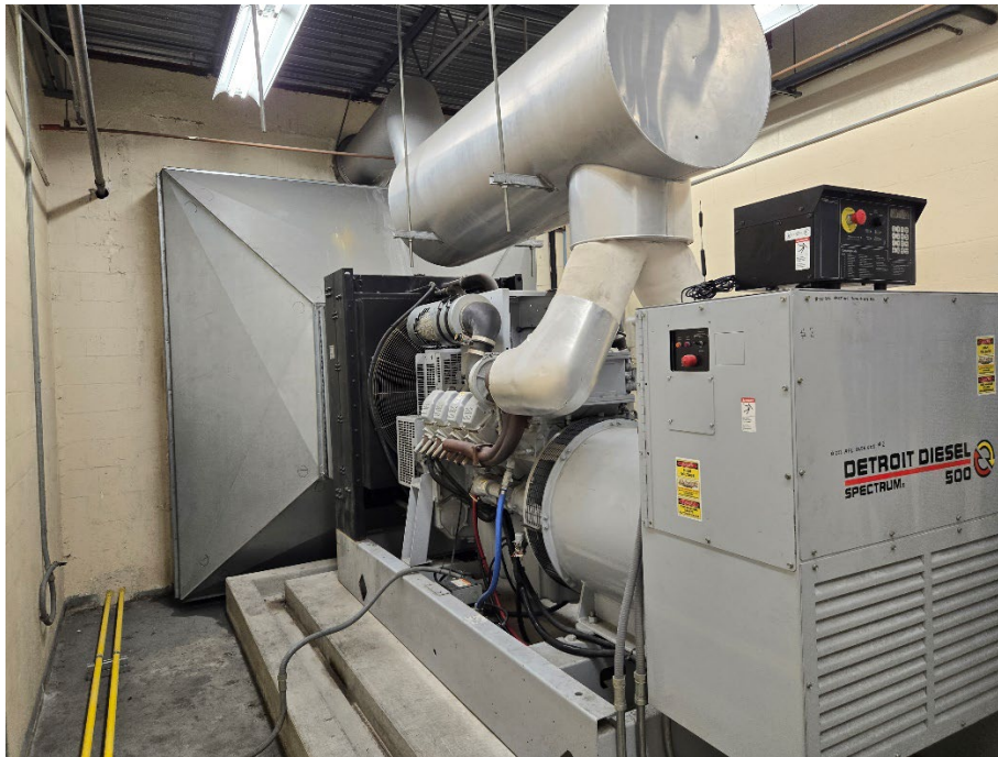
Figure 2.3 – Angled view of 500 KW generator
