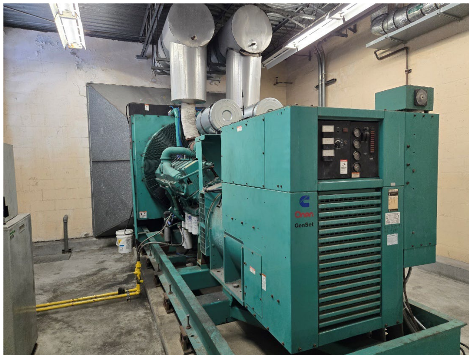
Figure 2.8 – 900 KW Generator Room (looking in from door)
