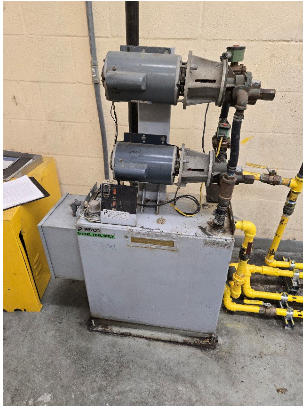
Figure 2.5 – Associated diesel day tank inside 500KW generator room
