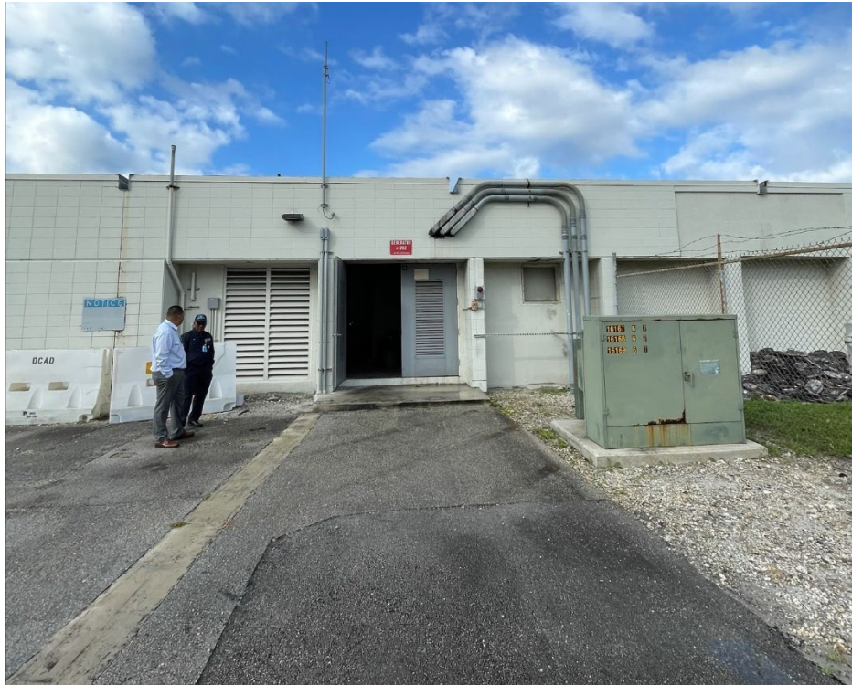
Figure 1.10 – Frontal view of entry doors into electrical room, pad mounted transformer, and overhead pipes leading inside
