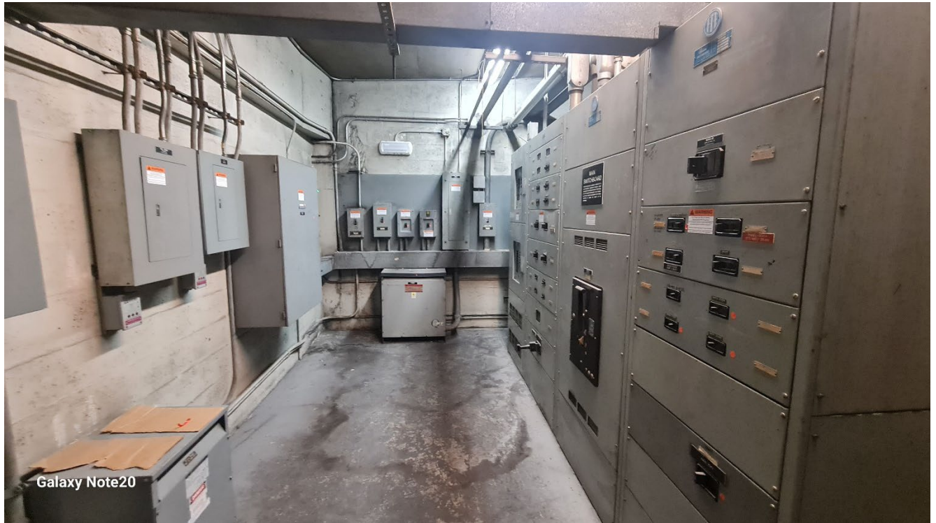
Figure 4.7 – Front side of switchgear, view of electrical room taken from entry door. South wall of electrical room on left side of photo.
