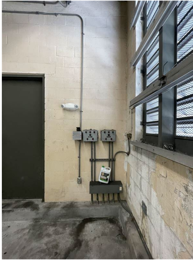
Figure 2.11 – Northeast corner of 900KW Generator Room
