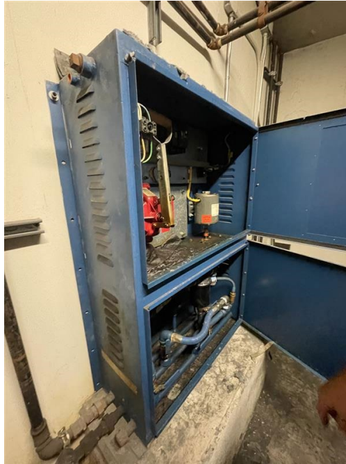
Figure 4.20 – Control device within diesel tank room
