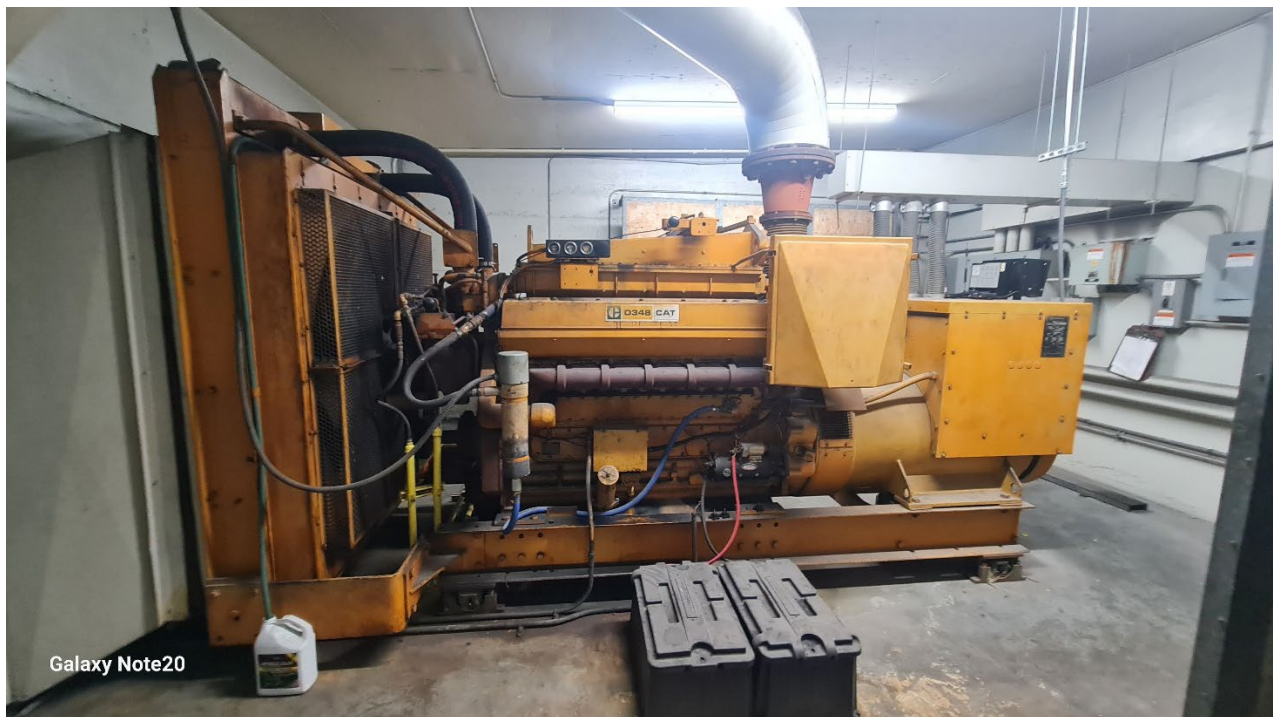
Figure 4.2 – POV from main doors/hallway looking into generator room (facing west)
