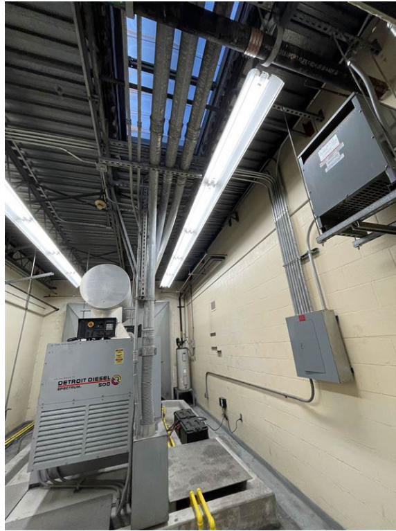
Figure 2.4 – Wide-angled view within 500 KW generator room
