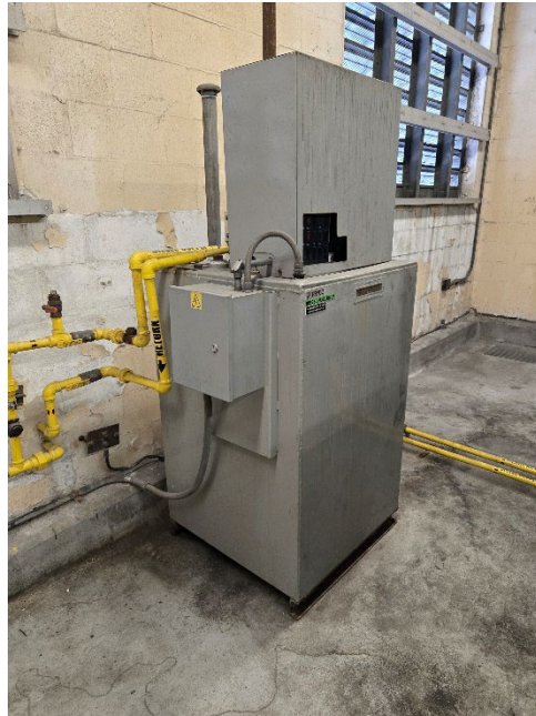
Figure 2.13 – Associated diesel day tank inside 900 KW generator room
