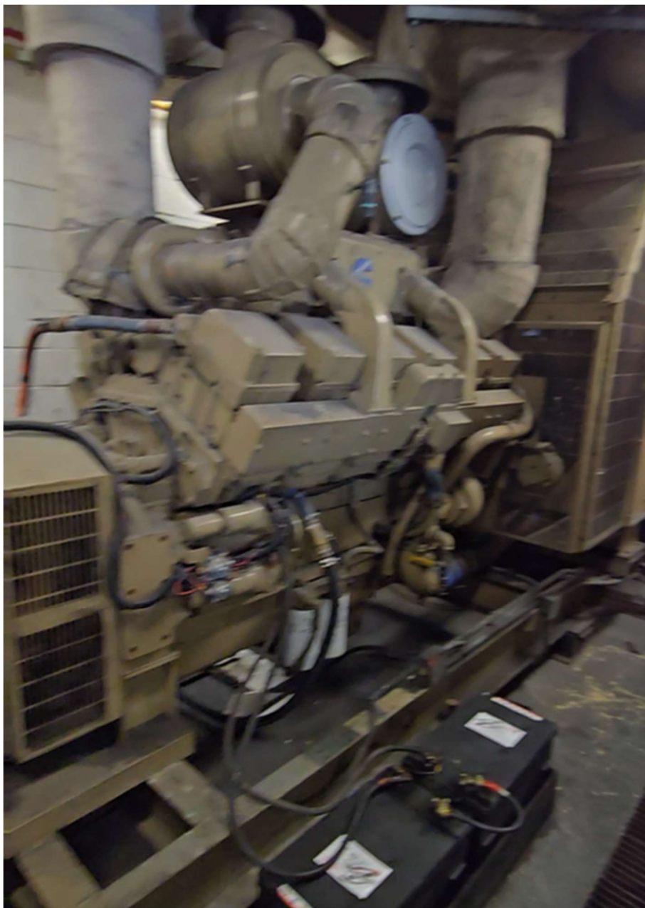
Figure 2.3 – 750 KW Generator #2 (Interior / East Plenum Location)
