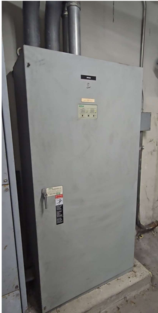
Figure 1.7 – Close up view of ATS #2
