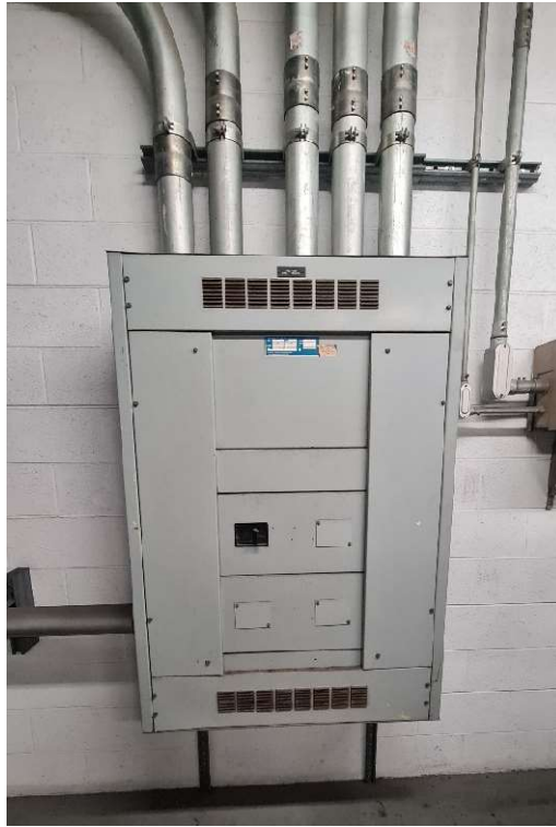
Figure 5.6 – Main emergency disconnect (GSB) frontal view
