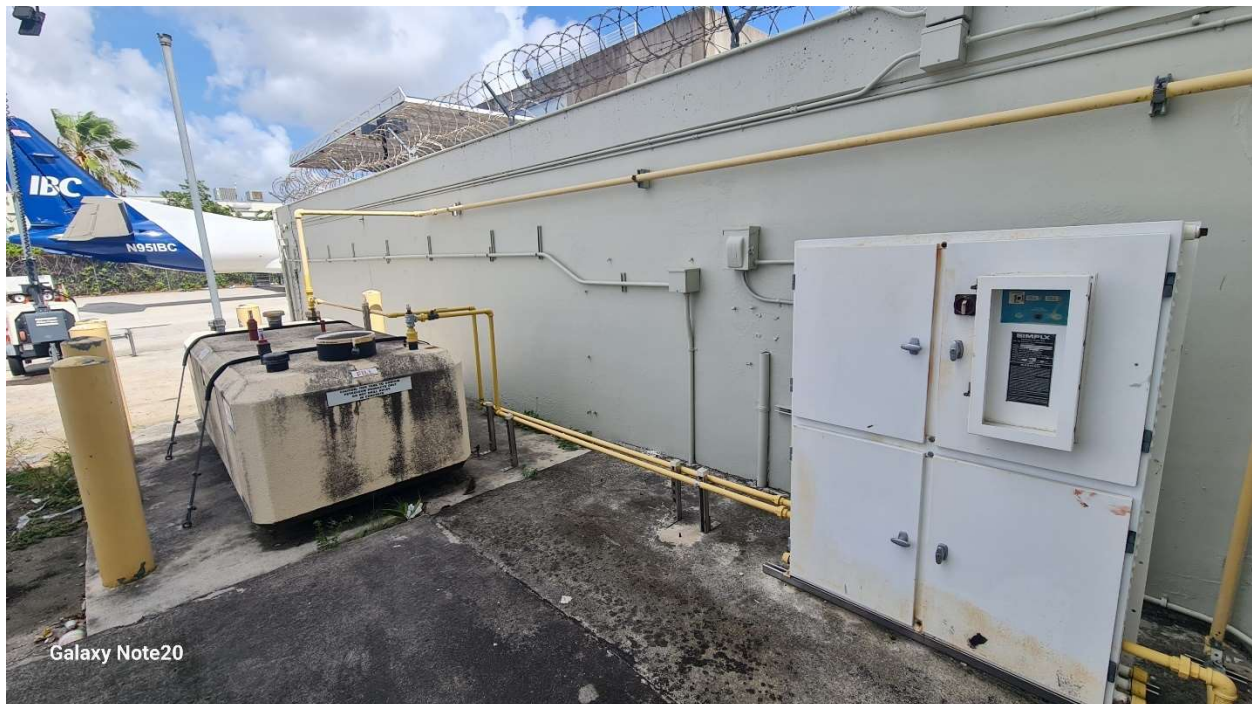
Figure 5.26 - Diesel tank system with equipment in vicinity. Airside.
