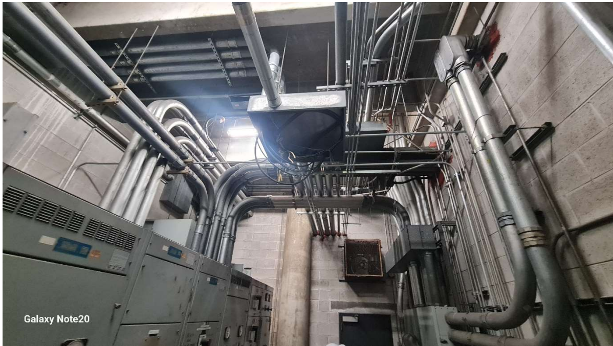
Figure 5.16 – Switchgear room aerial view of piping configuration from above
