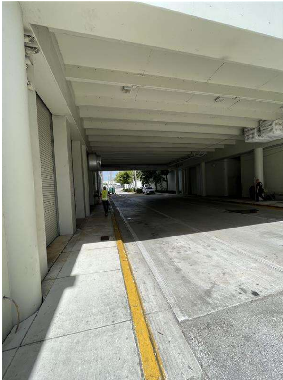
Figure 5.20 – Roadside view outside mechanical room doors, facing east. FPL vault and generator room to right of photo.
