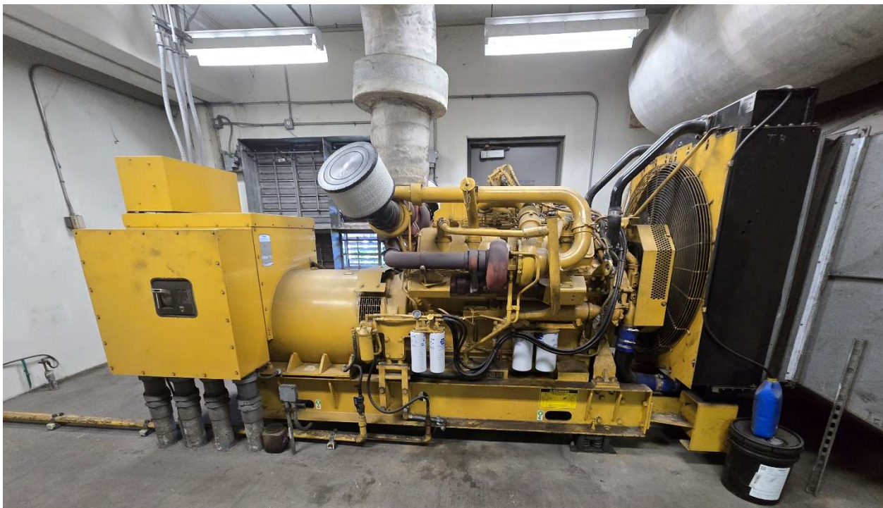
Figure 1.3 – 750kW generator (taken from interior entrance)
