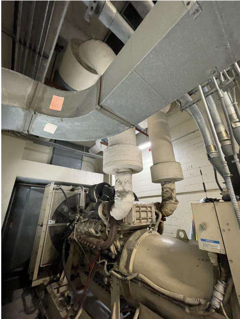
Figure 3.3 – Alternative frontal view of generator
