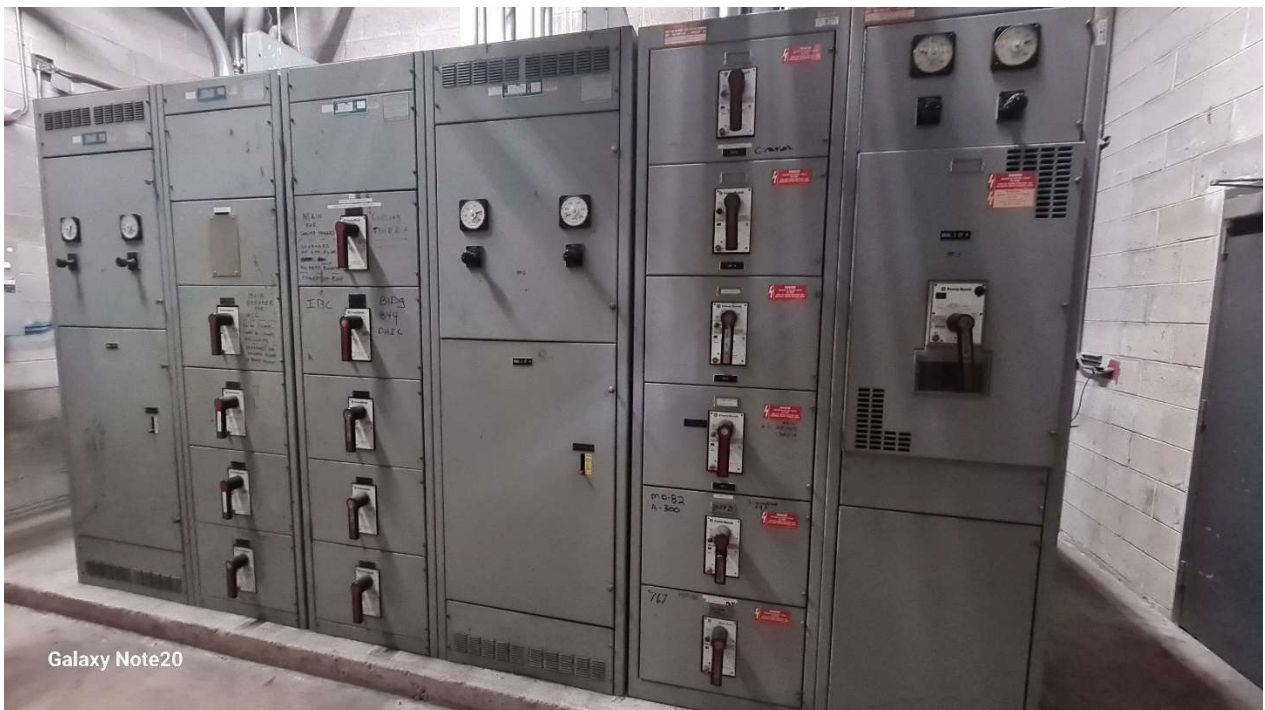
Figure 5.13 – Main switchgear unit
