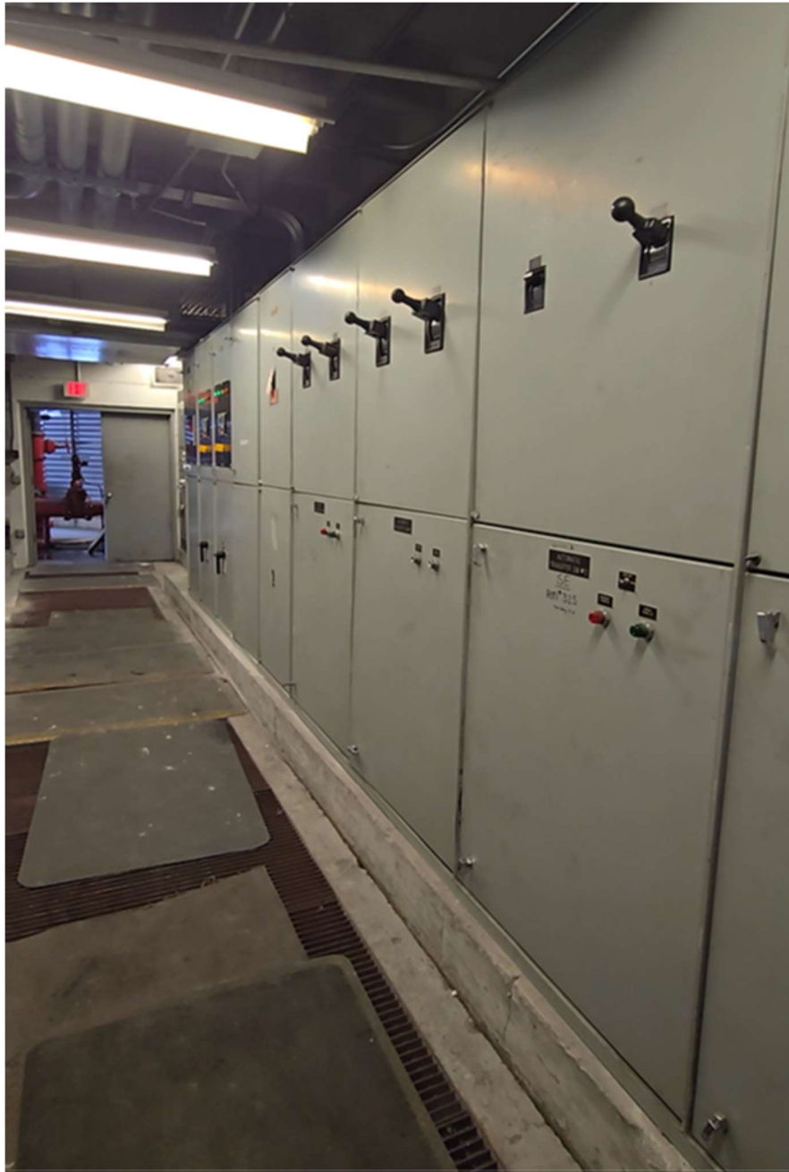
Figure 2.9 – Hallway of switchgear room, facing southwest. Major switchboards, panels, and switches to be replaced. Generator room behind doors in background.
