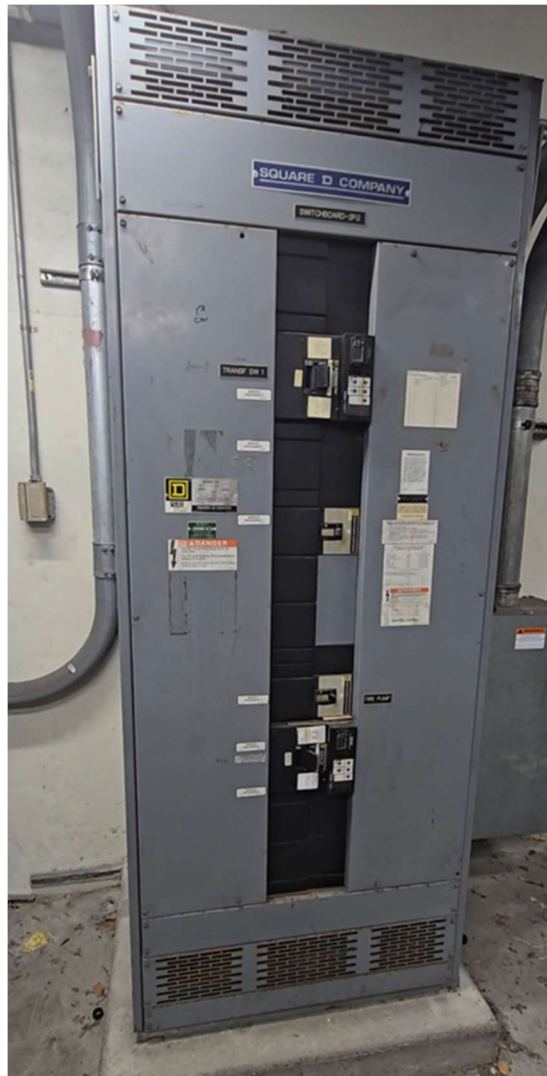
Figure 1.8 – Close up view of Switchboard 2FG
