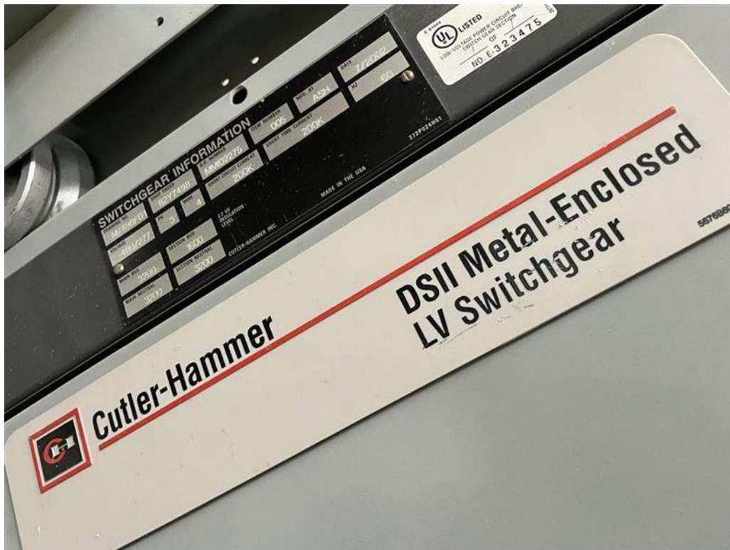
Figure 3.17 – Emergency Main in Switchgear Room. Entrance doors to left.
