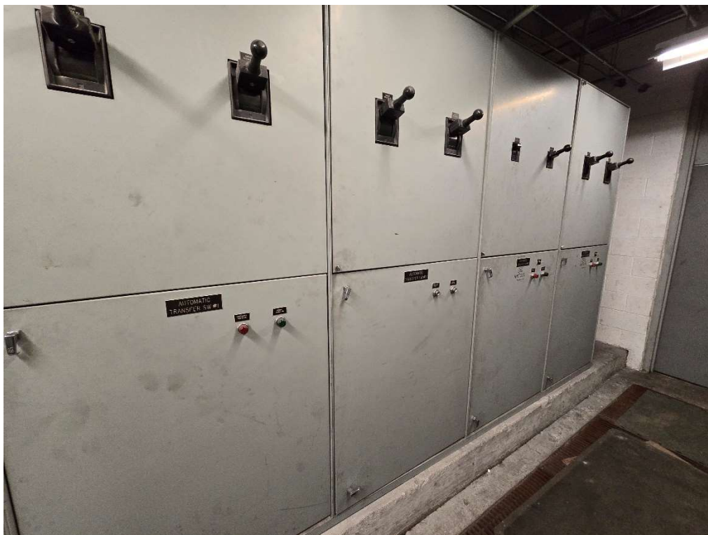
Figure 2.14 – Lineup of 4 ATS's. Located in NW corner of switchgear room towards interior, besides rear doors.
