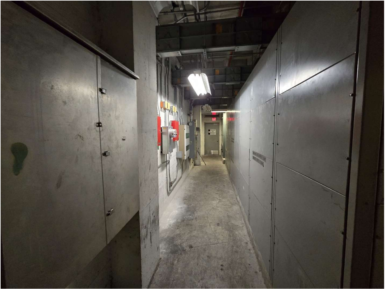
Figure 2.11 – Hallway behind main switchgear units on east side of switchgear room (located left of photo in Fig 2.10)
