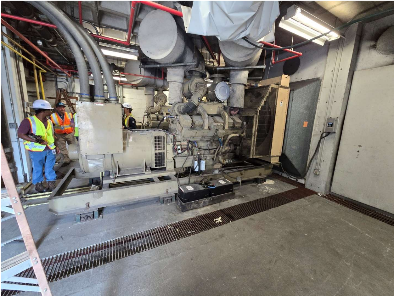
Figure 2.2 – 750 KW Generator #1 (Middle Plenum Location)
