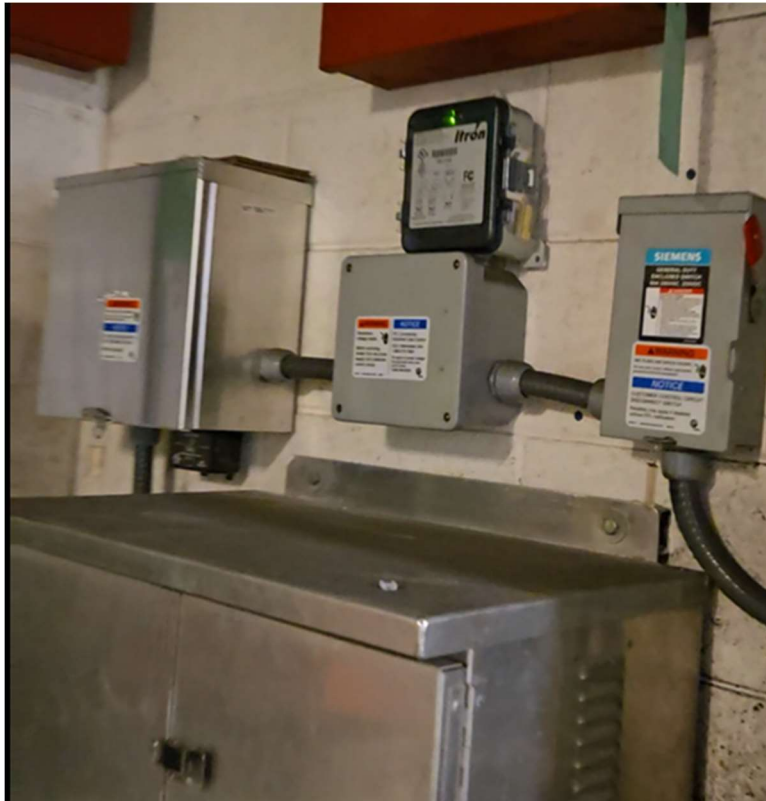
Figure 2.13 – CILC equipment found in southeast corner of switchgear room. Evidence for Tier 4 Generator requirement.
