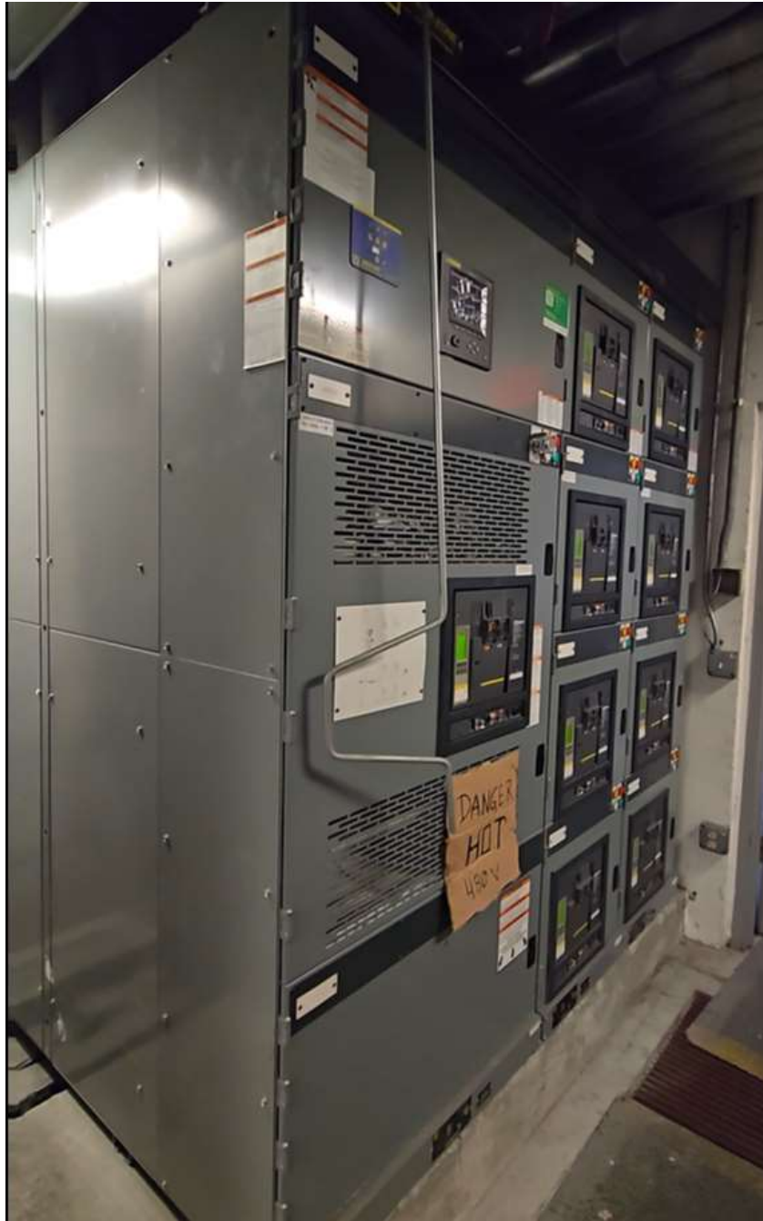
Figure 2.8 – Newer switchgear unit, found on SW side of switchgear room, adjacent to generator room doors. Connected to cable tray from FPL vault. This unit will not be replaced in scope.
