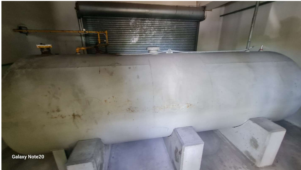
Figure 1.5 – 3000-gallon interior diesel tank with roll-up door in background
