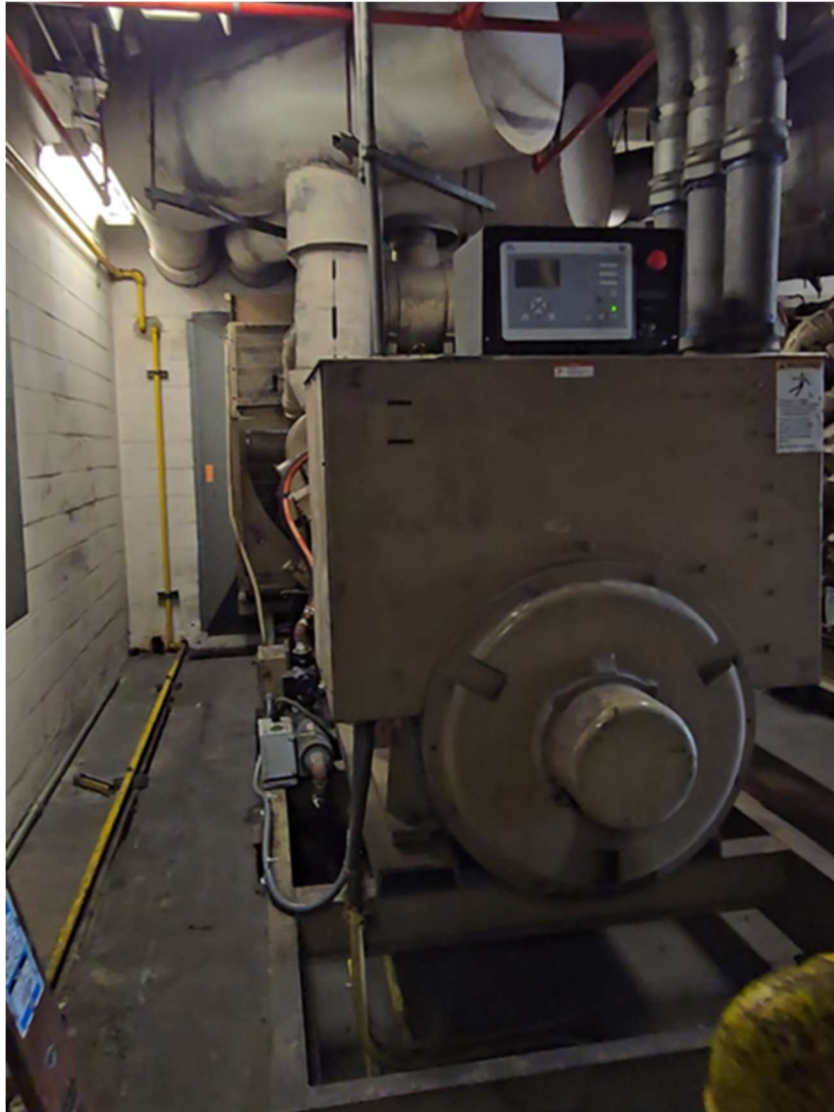
Figure 2.5 – Generator #2, taken from west of unit.
