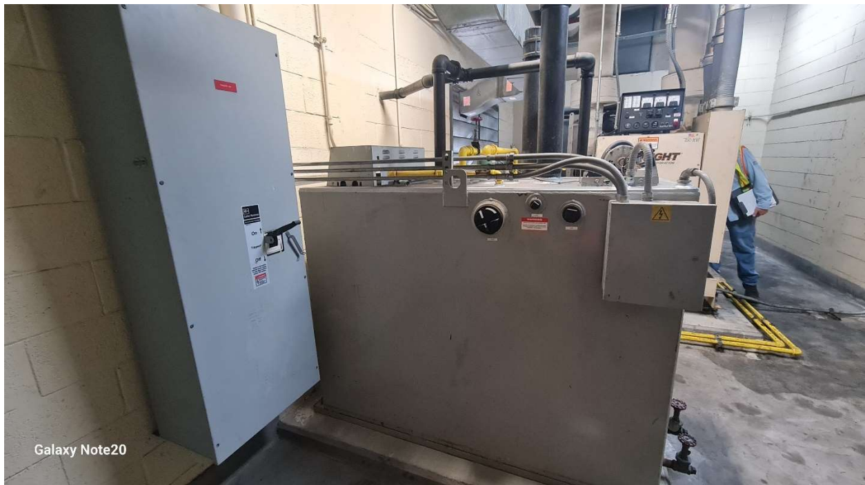
Figure 4.5 – Diesel tank and breaker in Room 214. Generator in back.
