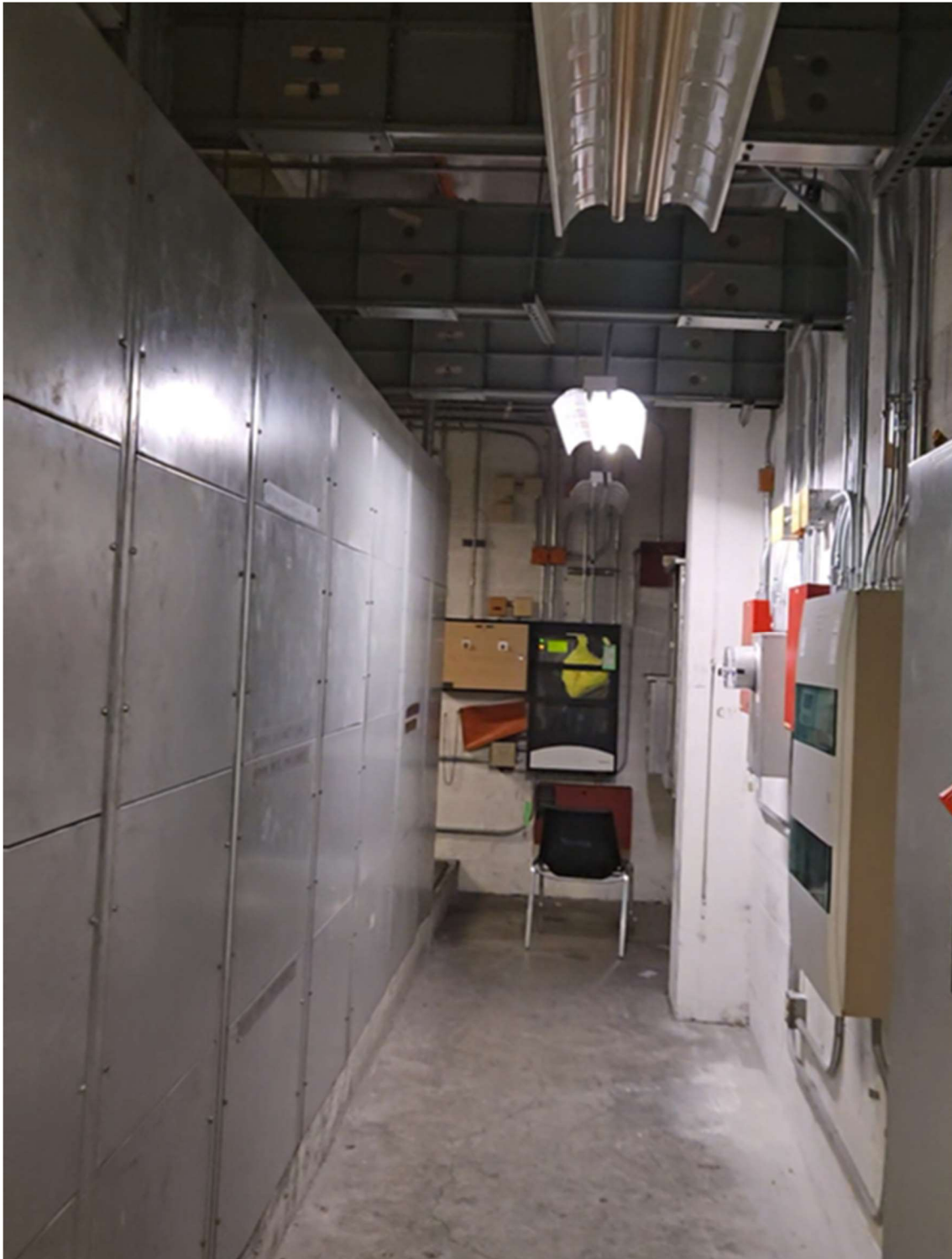
Figure 2.12– Hallway behind main switchgear units on east side of switchgear room, facing northeast (opposite end POV from Figure 2.11). 5 bus duct and 1 cable tray found overhead from FPL vault behind right wall.
