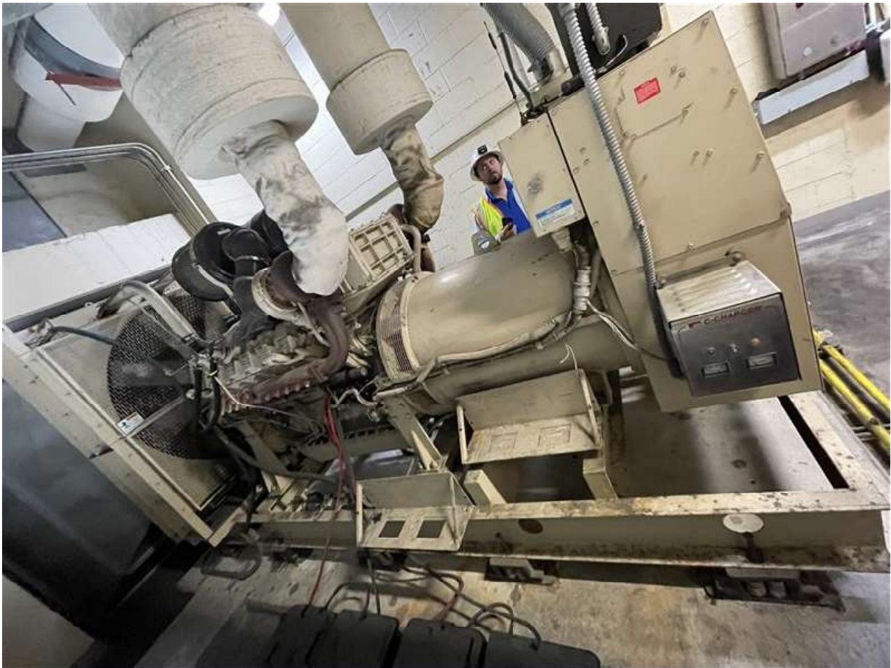
Figure 2.2 – Side view of generator
