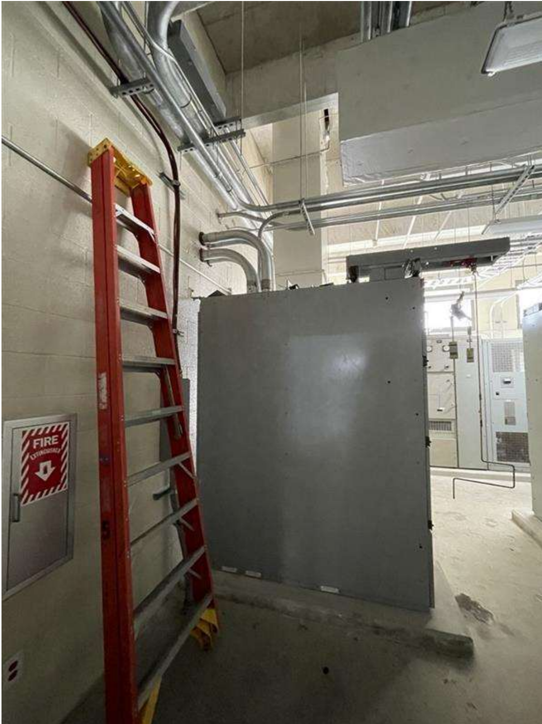
Figure 3.16 – Emergency Main Switchgear in Switchgear Room. Side view.
