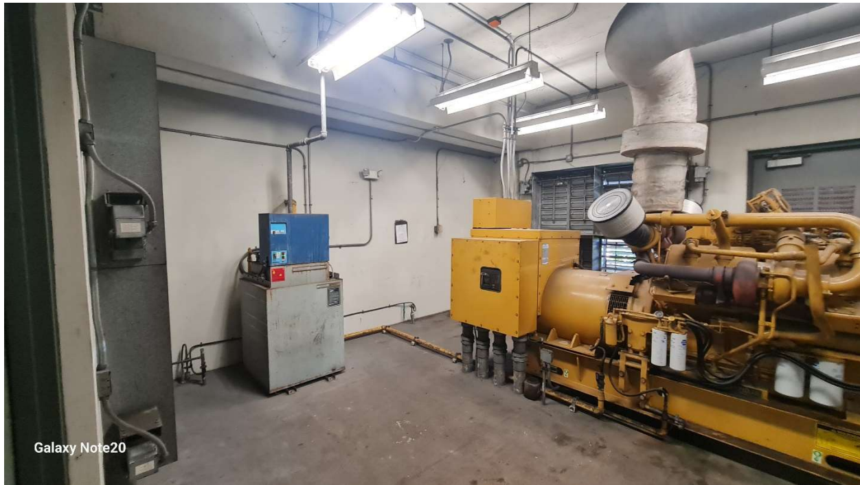
Figure 1.5 – Angled view of generator room
