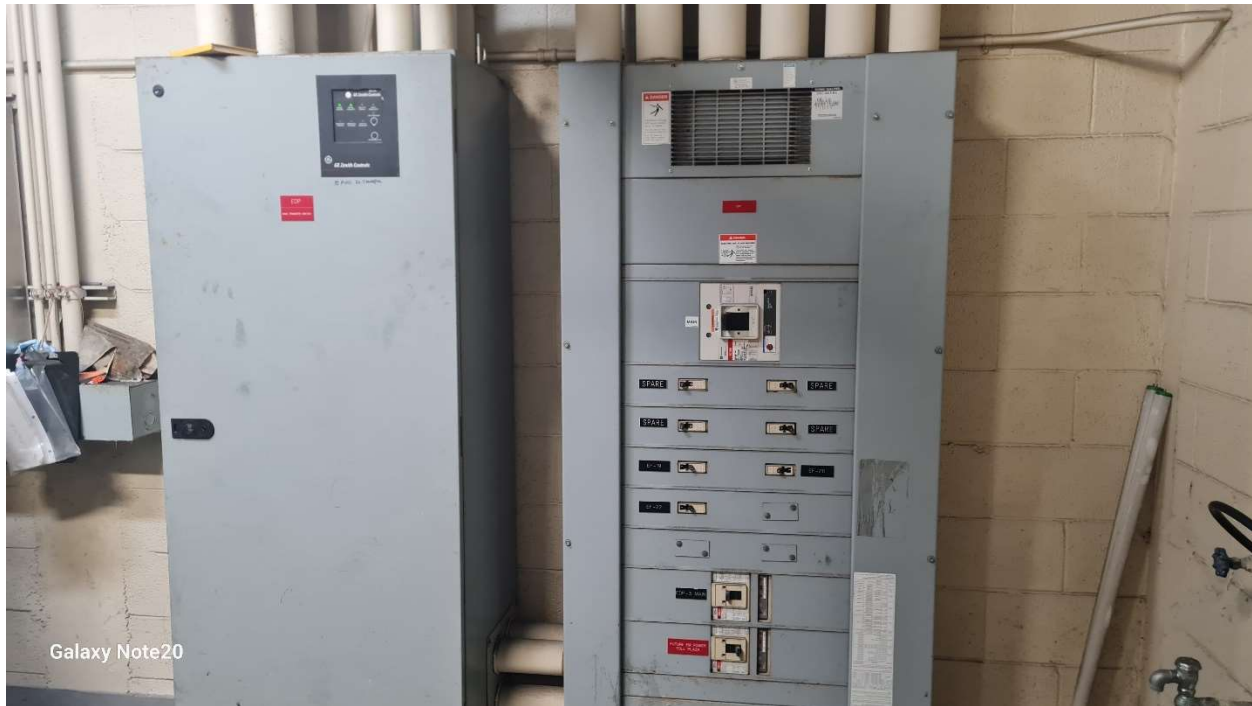
Figure 3.8 – 1000A Panel EDP with the ATS located on left. West wall of room.
