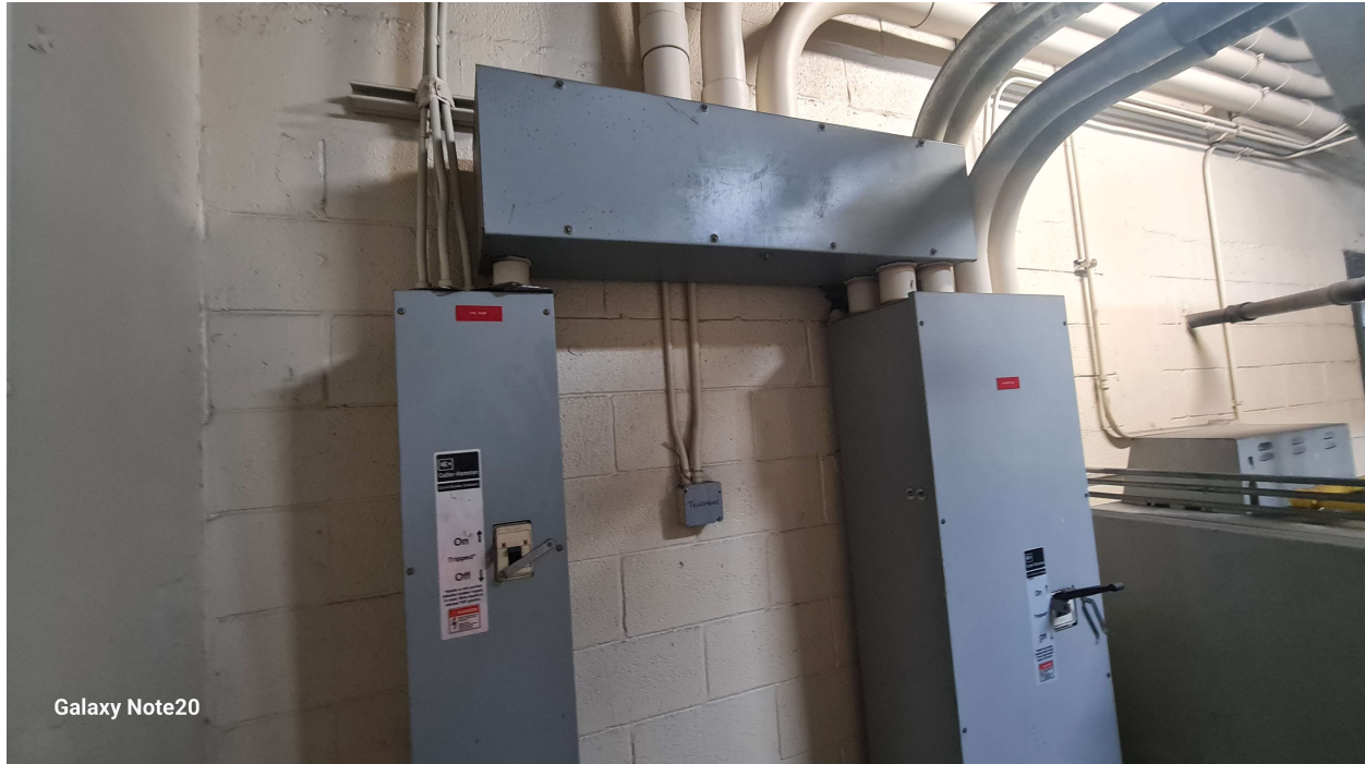
Figure 6.7 – Cable tray, 400A circuit breaker for fire pump and associated piping. East wall of room.
