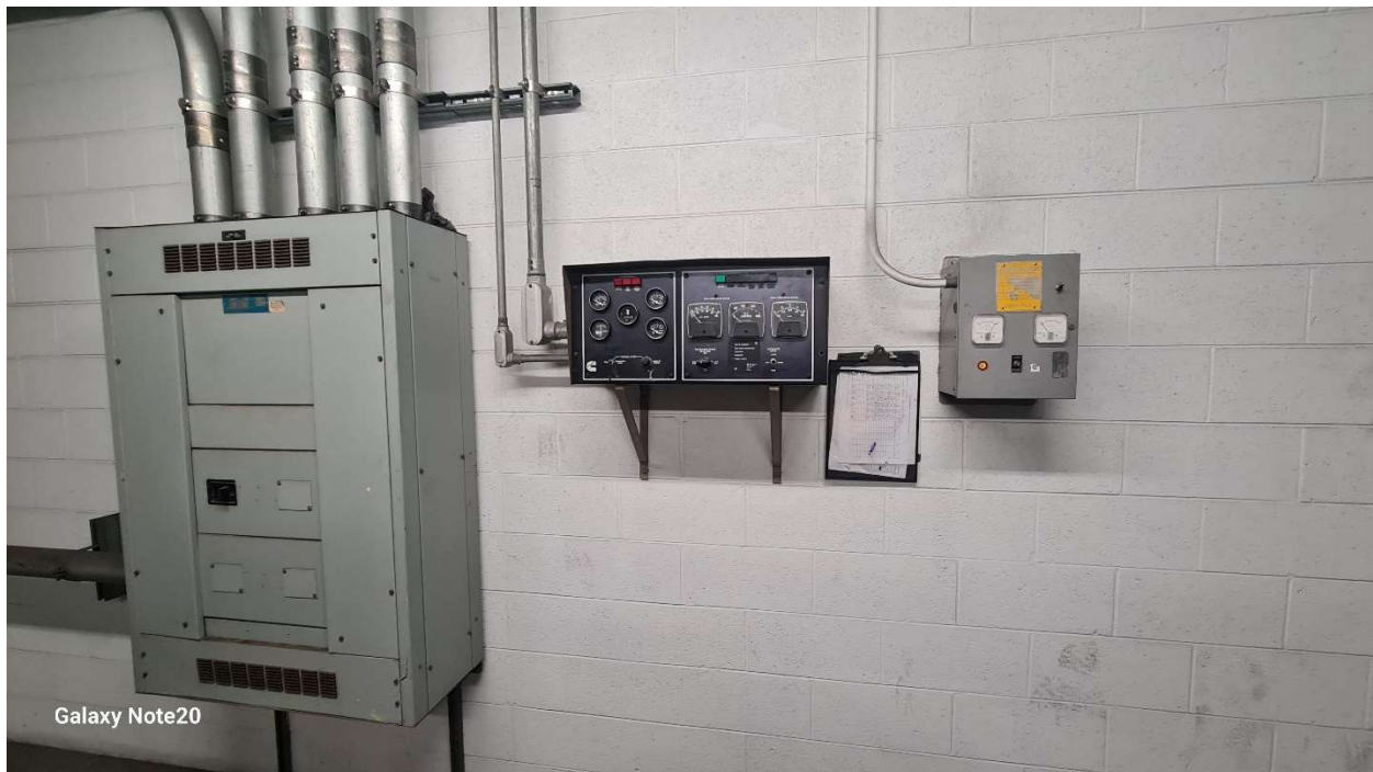
Figure 5.5 – Main emergency disconnect (GSB) and analog setup on west wall of generator room.
