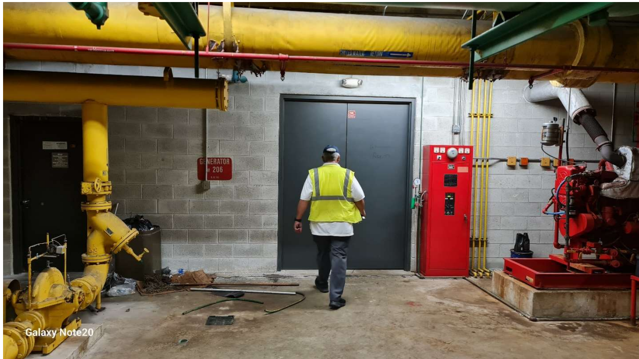
Figure 5.21 – Mechanical room view to doors leading into generator room (2 nd floor)
