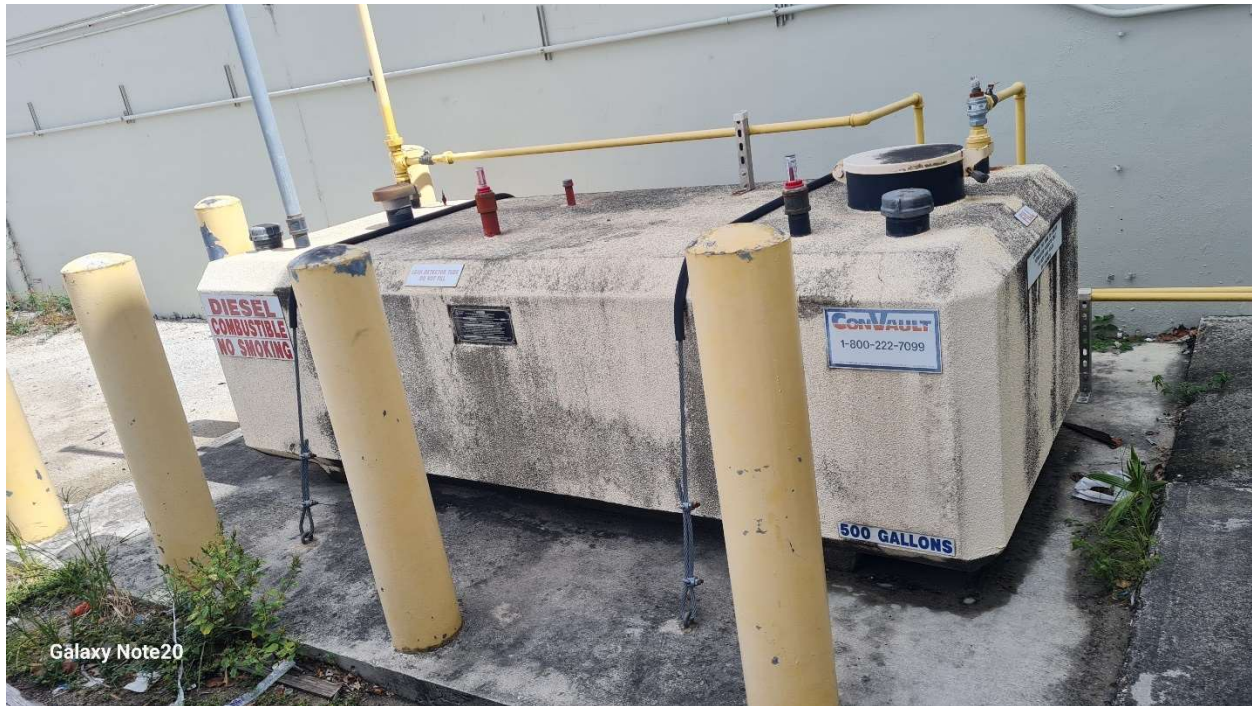
Figure 5.25 – 500-gallon diesel tank
