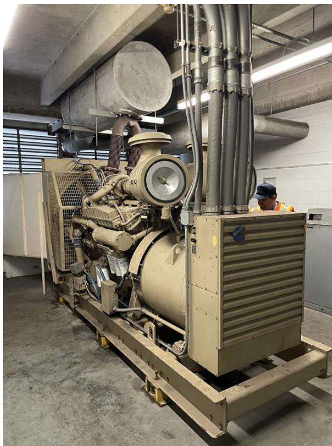
Figure 5.2 – Side of angle of generator
