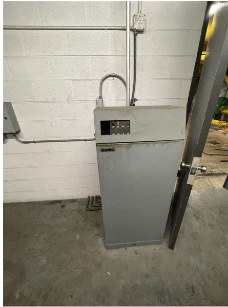
Figure 5.10 – Day tank for adjacent fire pump. Beside main entrance doors.
