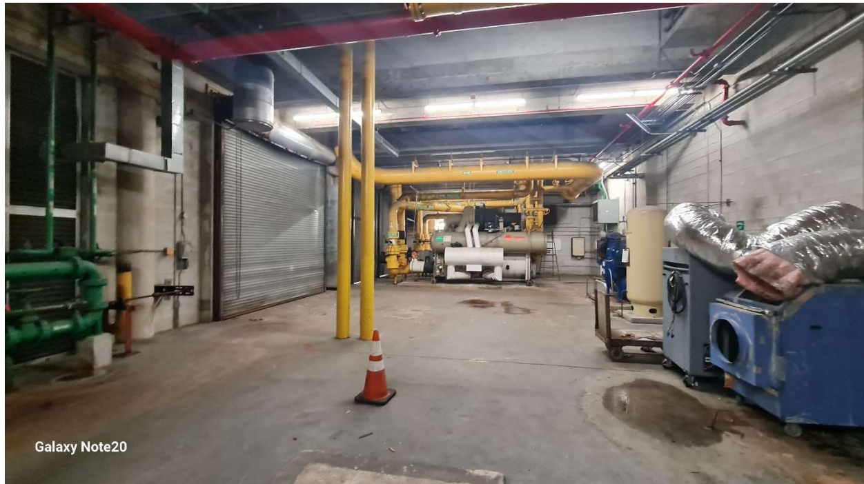
Figure 5.23 – Mechanical room, adjacent to switchgear room. Exit doors to outside on left.
