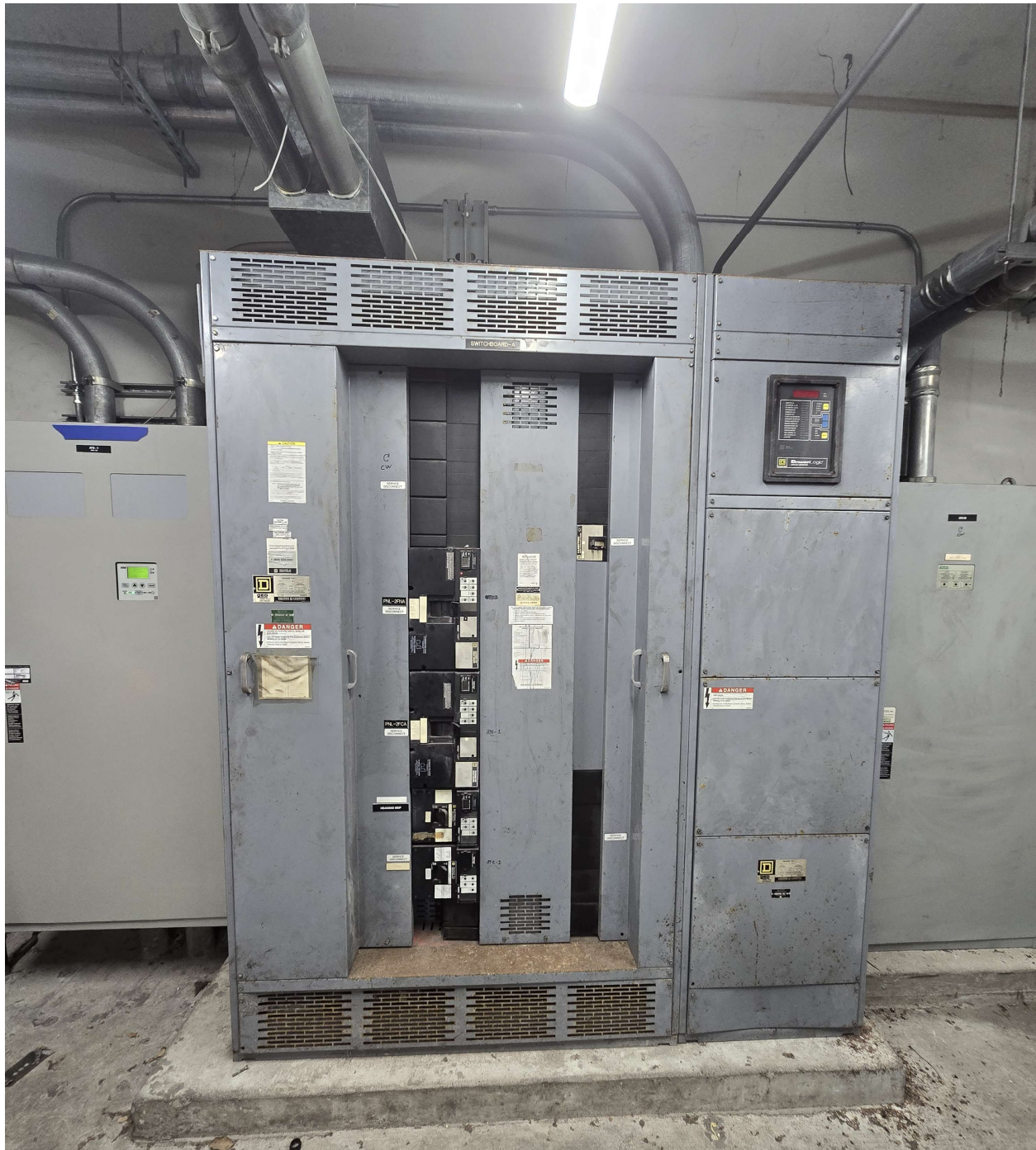
Figure 1.6 – Switchboard A, on north wall of electrical room. Flanked by ATS #1 (Left) & ATS #2 (Right).
