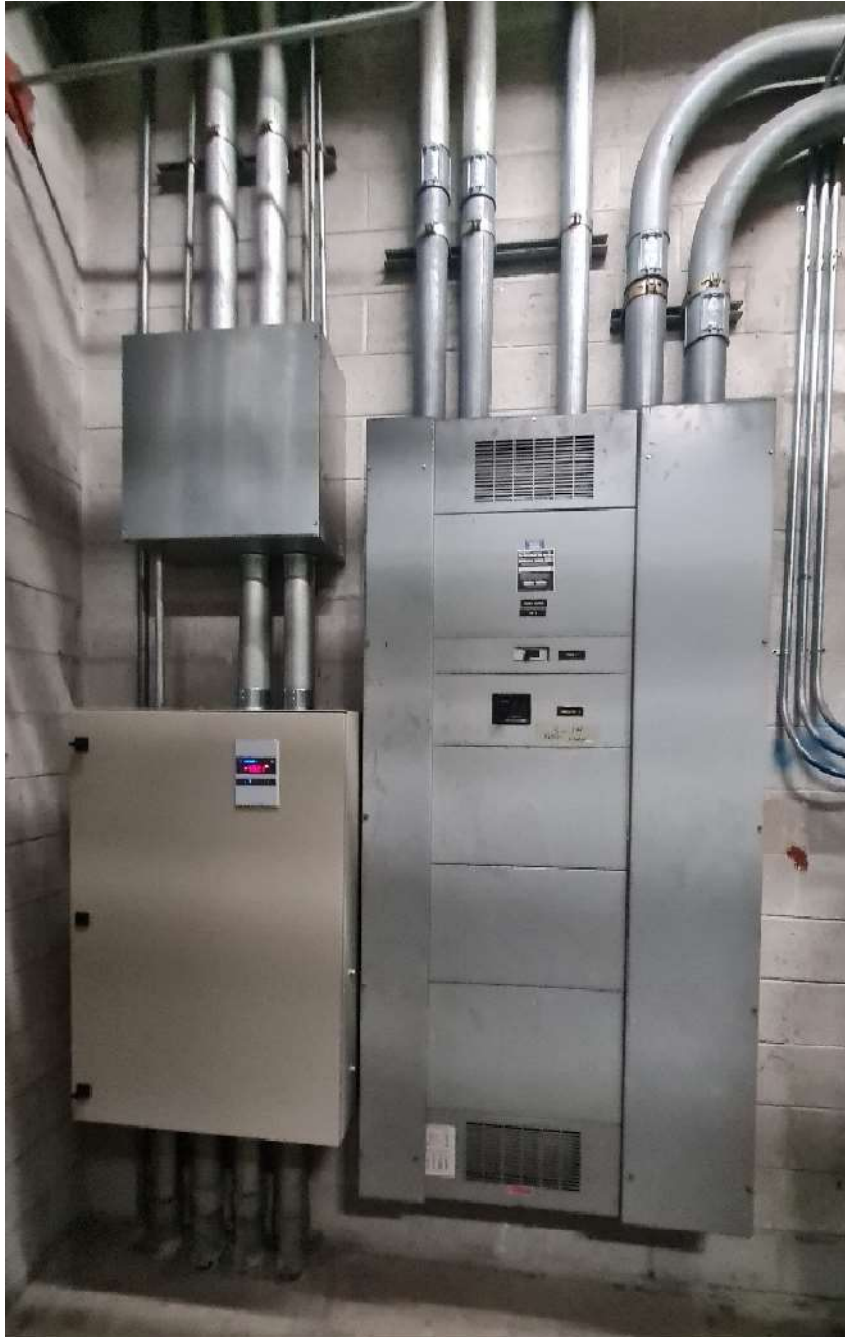
Figure 5.17 – Generator ATS & panel in southwest corner of switchgear room.
