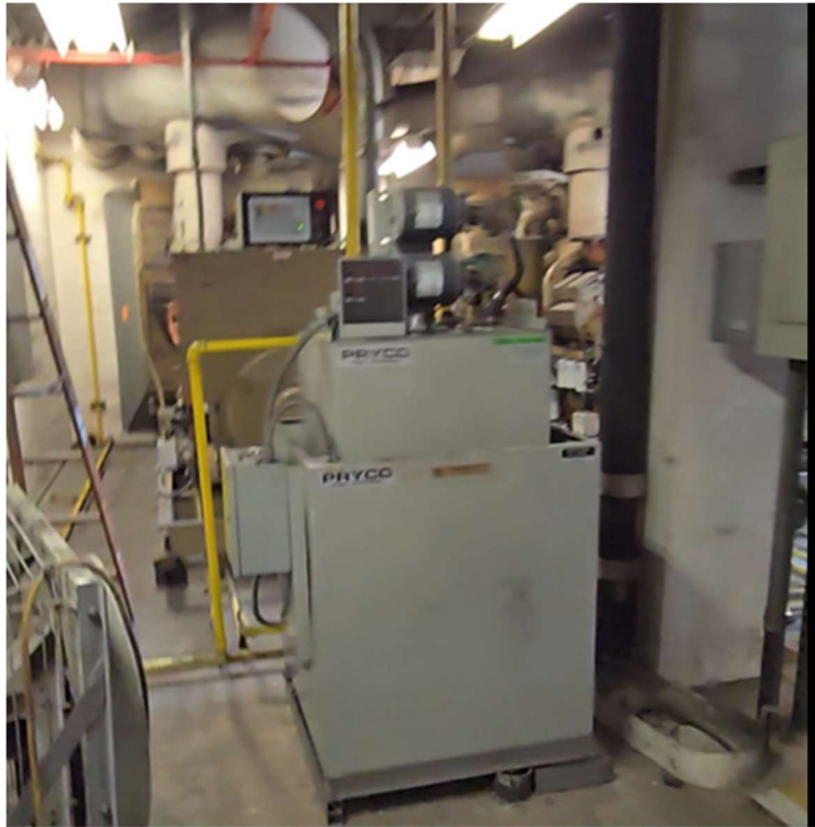
Figure 2.6 – Diesel day tank associated with Generator #2 (in back)
