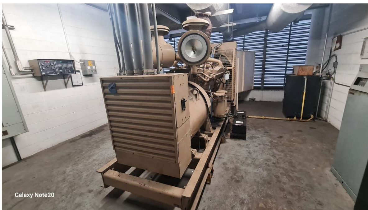
Figure 5.3 – Frontal view of generator with adjacent day tank and analog monitoring setup
