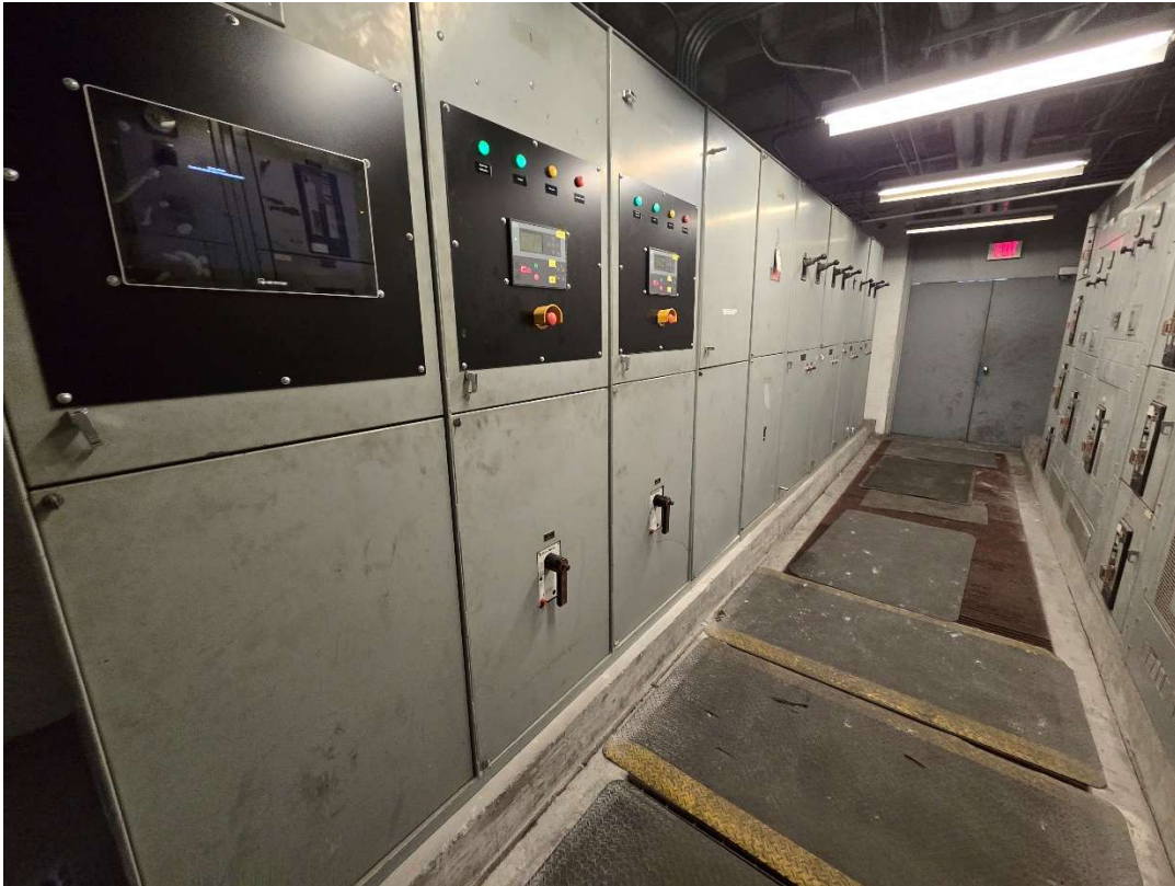
Figure 2.15 – Additional photo of main panel/ generator monitoring lineup in switchgear room, facing northeast (interior)
