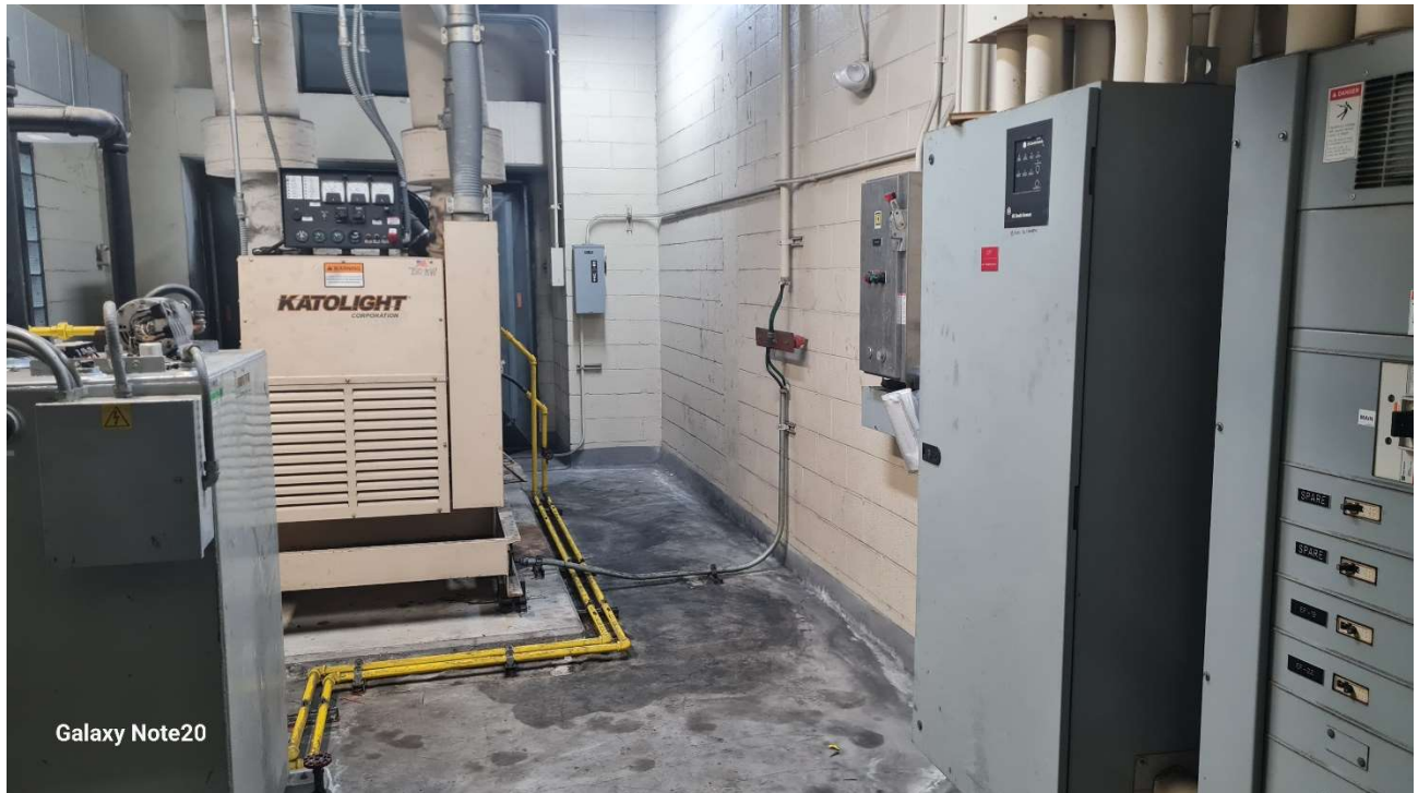
Figure 5.6 – Diesel tank to left, generator in back, EDP and ATS found on right
