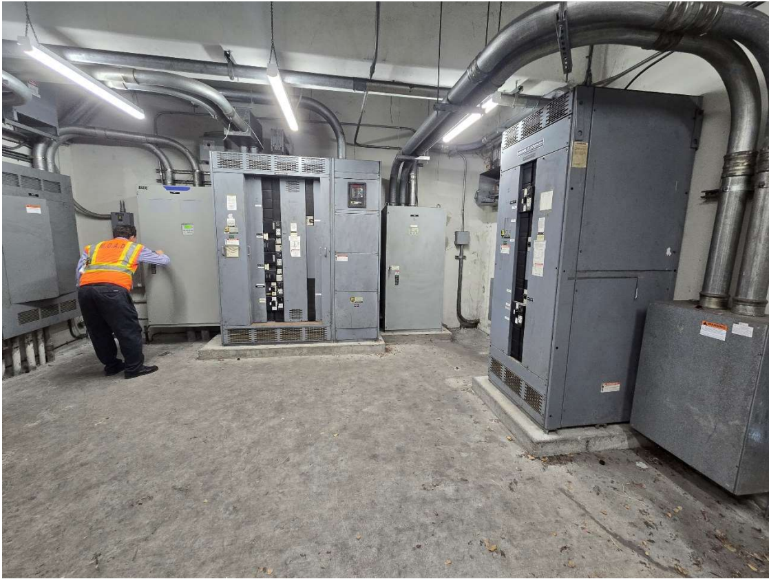
Figure 1.9 – Wide-panned view of electrical room, facing north. Switchboard A, ATS #1 & 2 on north wall. Switchboard 2FG on right. Downstream panels on left and to left of photo.
