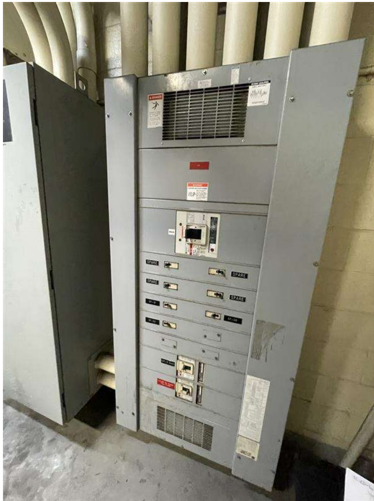
Figure 3.9 – 1000A Panel EDP with the ATS located on left. Expanded view.
