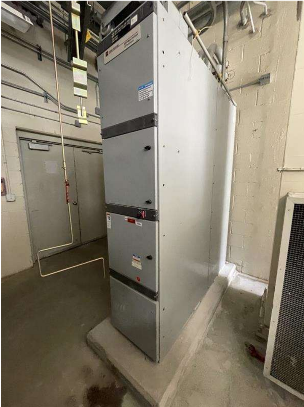
Figure 3.15 – Emergency Main Switchgear in Switchgear Room. Entrance doors to left.
