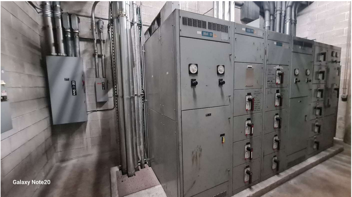
Figure 5.12 – Frontal side view of vertical conduit run, main switchgear unit, and Main #4 on left (serving fire station)
