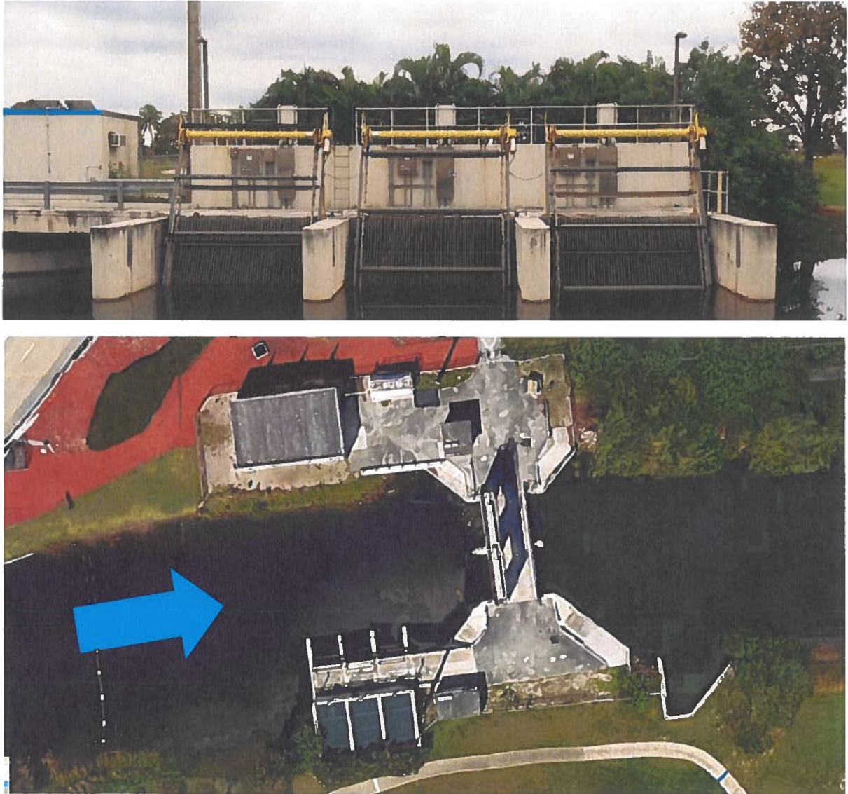
Figure 3: Structure S-25B Forward Pump – Upstream and Aerial View
