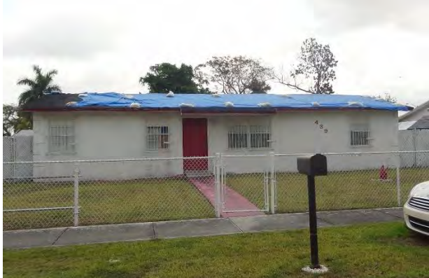
Figure 7: Unrepaired roofs pose a safety risk
