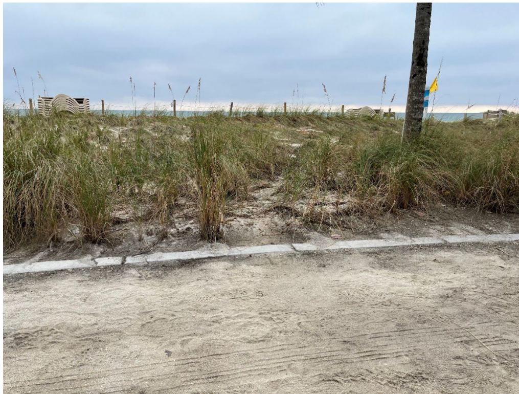
Figure 5: Photo facing shore perpendicular of the Miami-Dade County Main Segment (Bal Harbour) (R-30) showing flattened dune vegetation from wave overtopping on 17 November 2022.
