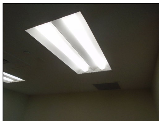
Courthouse Interior Lighting 3
