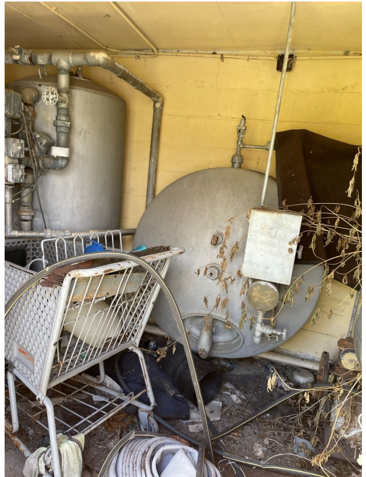
Interior of Dining Hall maintenance shed with end of tank through wall.
