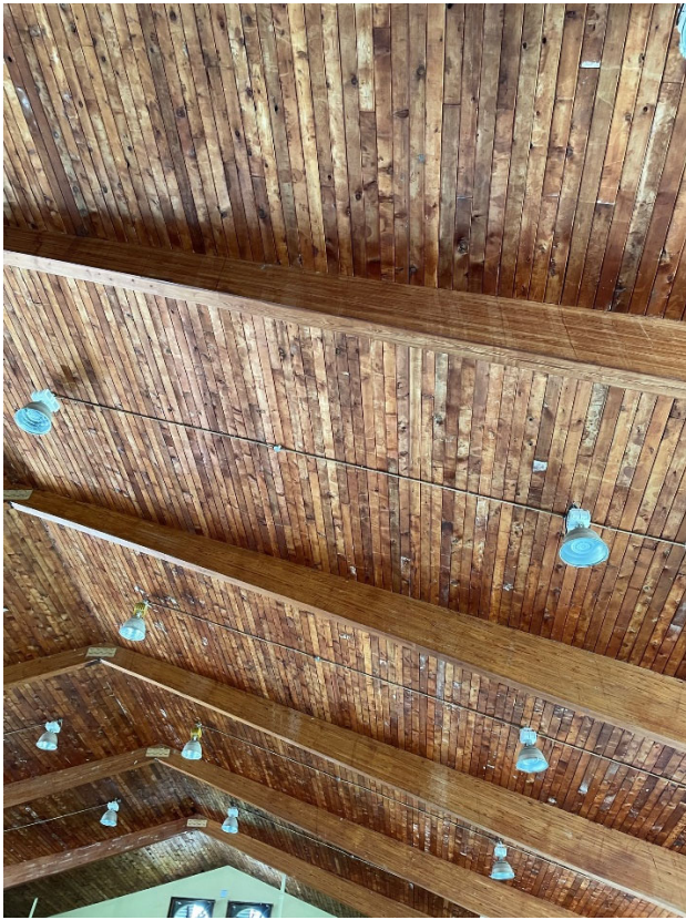
Close-up view of arched trusses, light fixtures, and tongue and groove roof decking.
