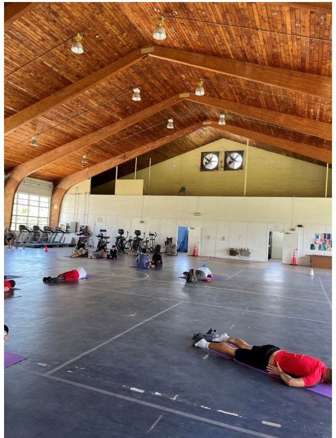
Indoor view of main gym with arched trusses and tongue and groove roof decking.
