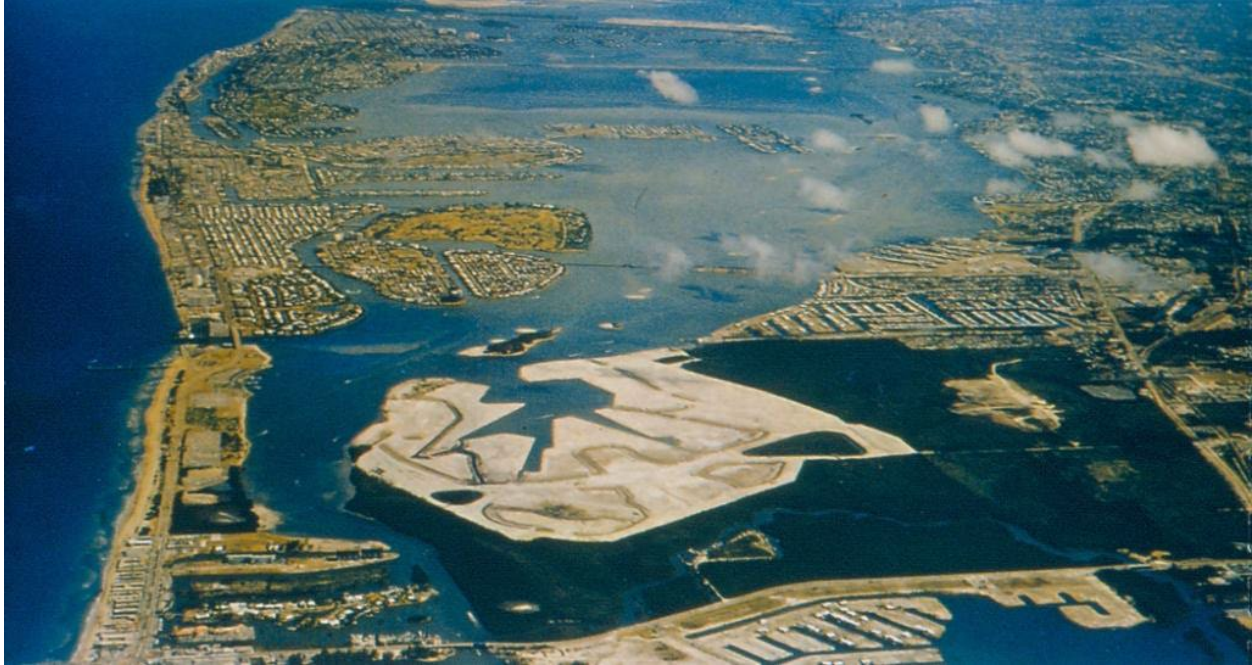
Land filling and grading of the Interama site, North Miami, c. 1964. Aerial photo, c. 1964. Courtesy HistoryMiami Museum
