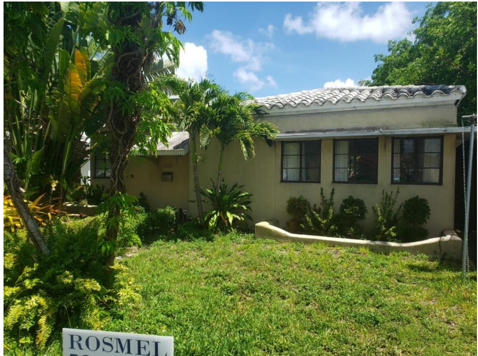
View from the street front of the subject property, showing the façade windows proposed for replacement, May 2020.
