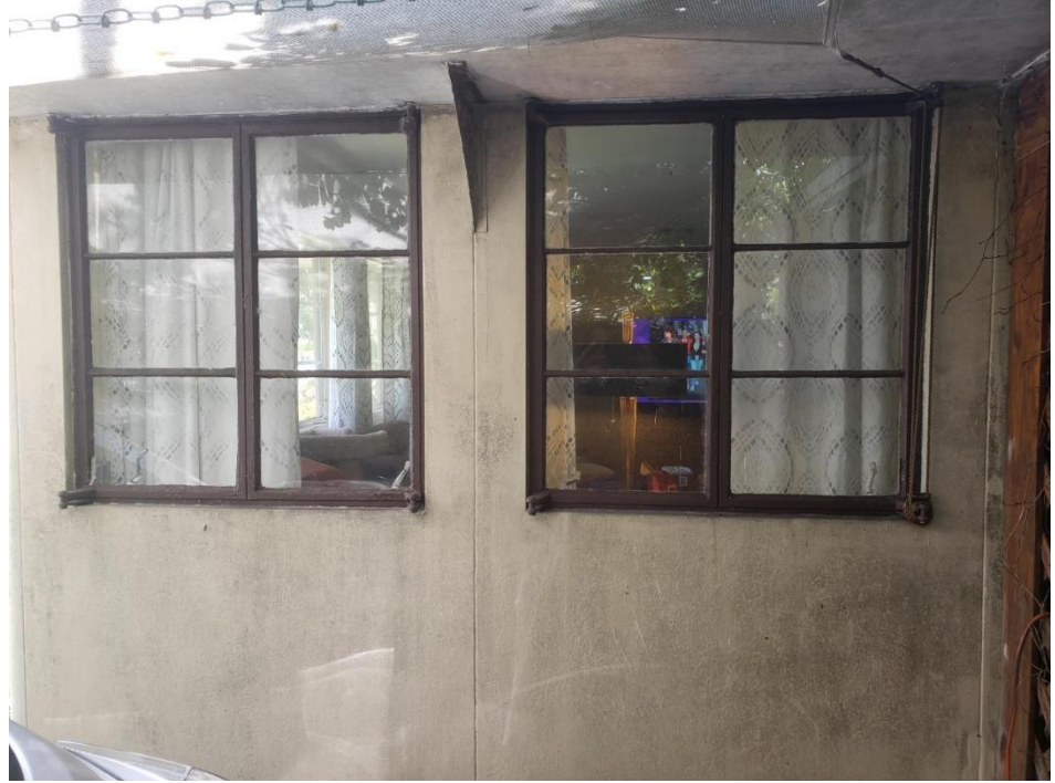
Original casement windows (not the façade, but illustrative of the façade windows), May 2020.
