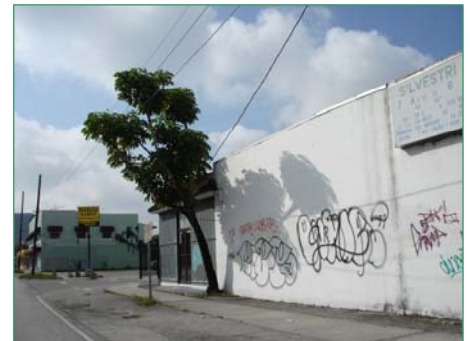
Invasive exotic tree, too close to building and power lines
