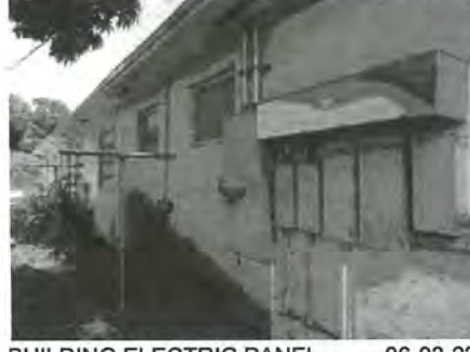
BUILDING ELECTRIC PANEL
