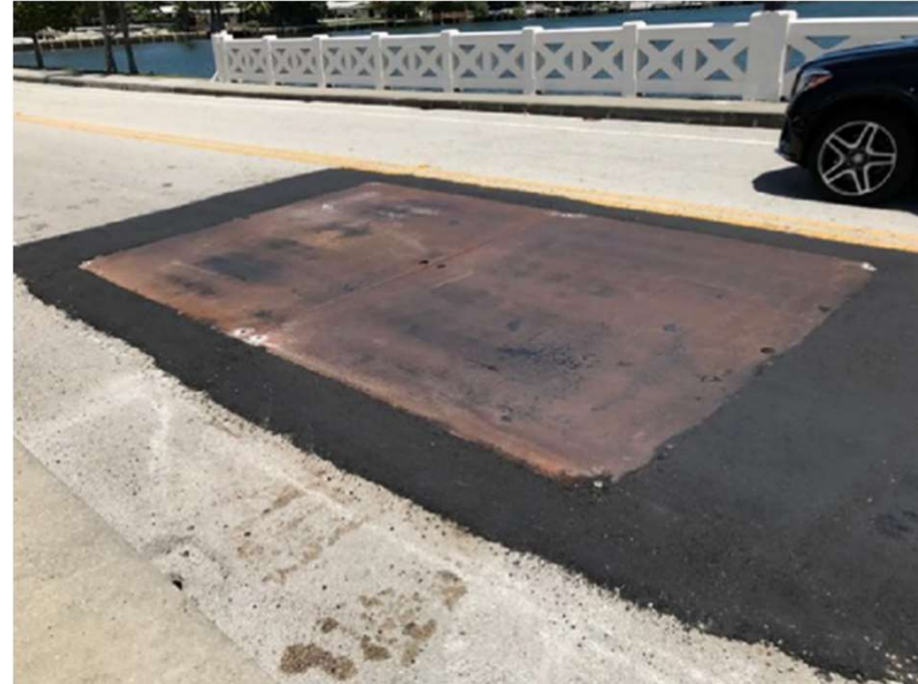
Right: Steel plate covering deck failure
