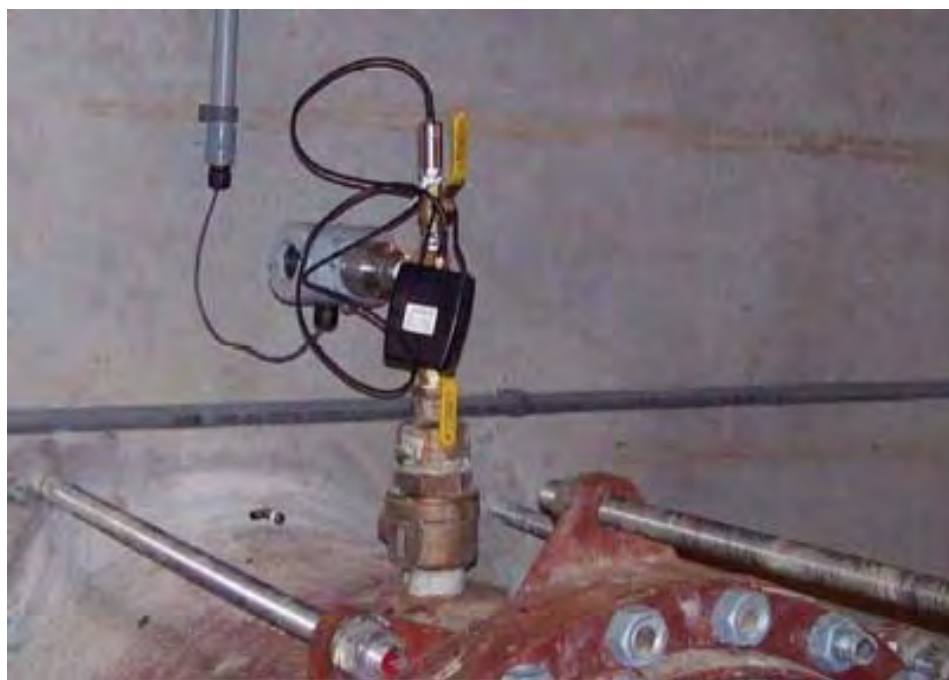
Figure 6-1 - Example Pressure Logger Installation
